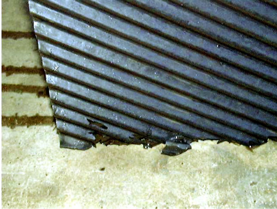
Figure 2.2-6. Location B, damaged coalescing plate.
