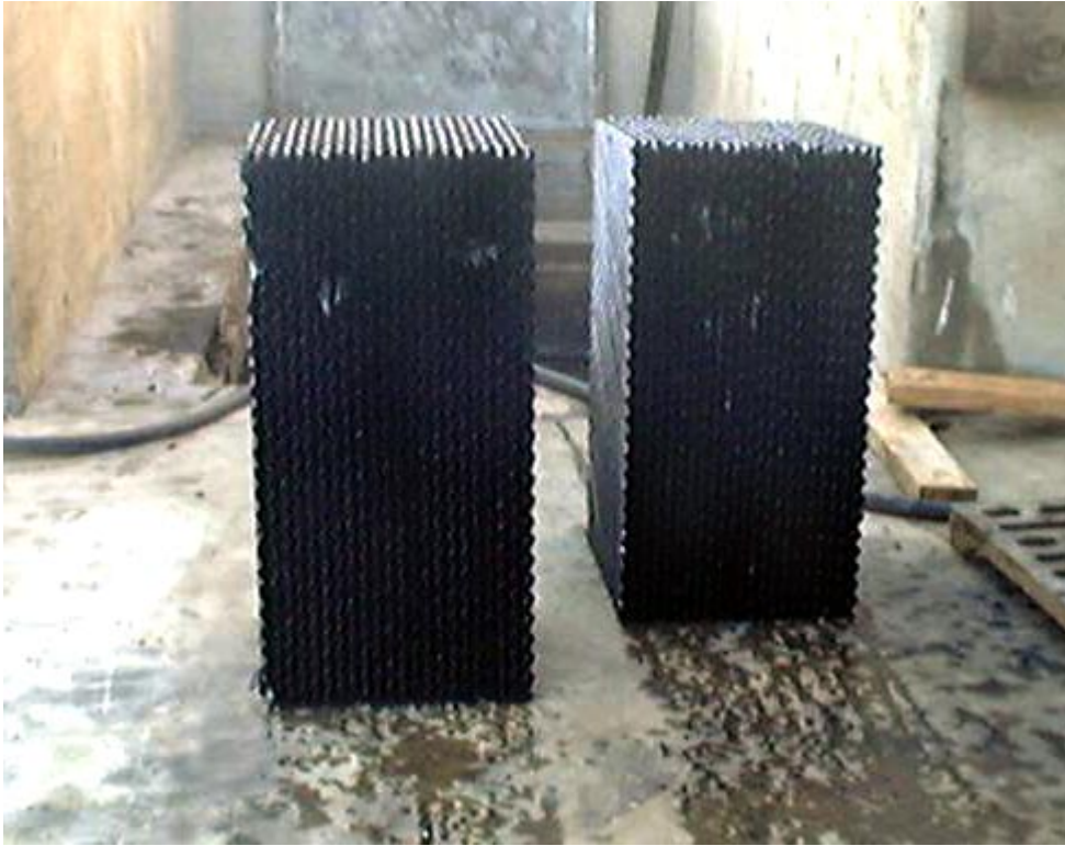
Figure 2.2-4. Location B, coalescing plate packages removed for cleaning.
