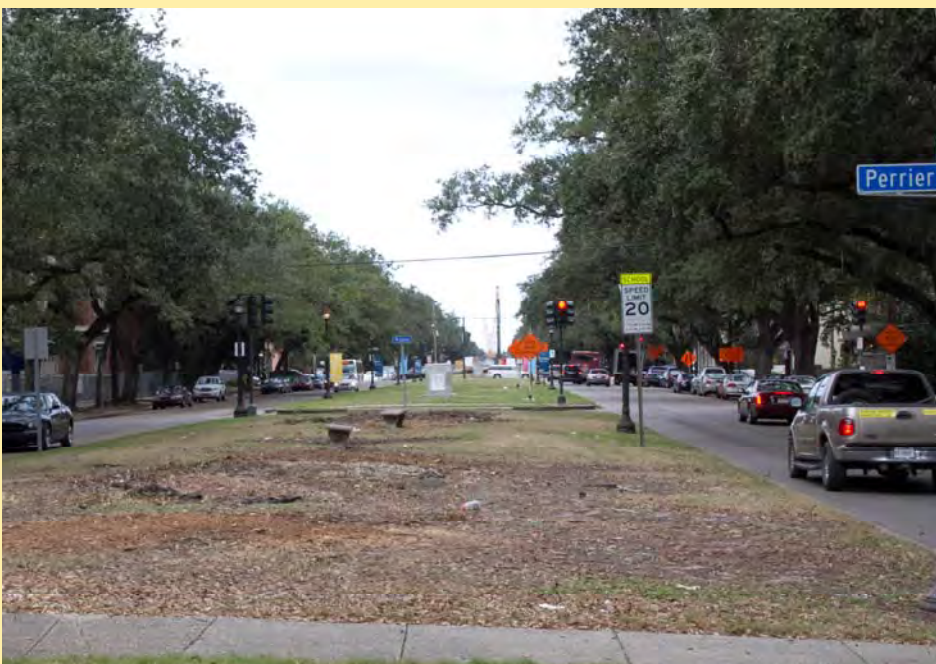
This recent photo of Napoleon Avenue at Perrier Street shows shrub clearing work is underway as part of SELA Phase III. USACE Photo by Scott Riecke
