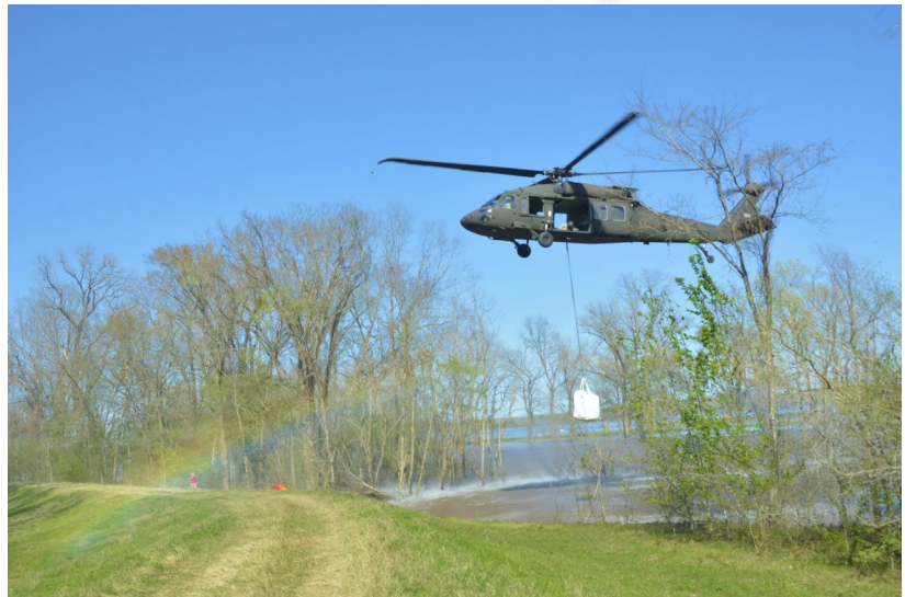
March 17 - A National Guard helicopter placed super-sized sandbags in the East Point Levee (along Loggy Bayou, which forms the Bossier-Red River River Parish line), which eroded because of rushing floodwaters.
