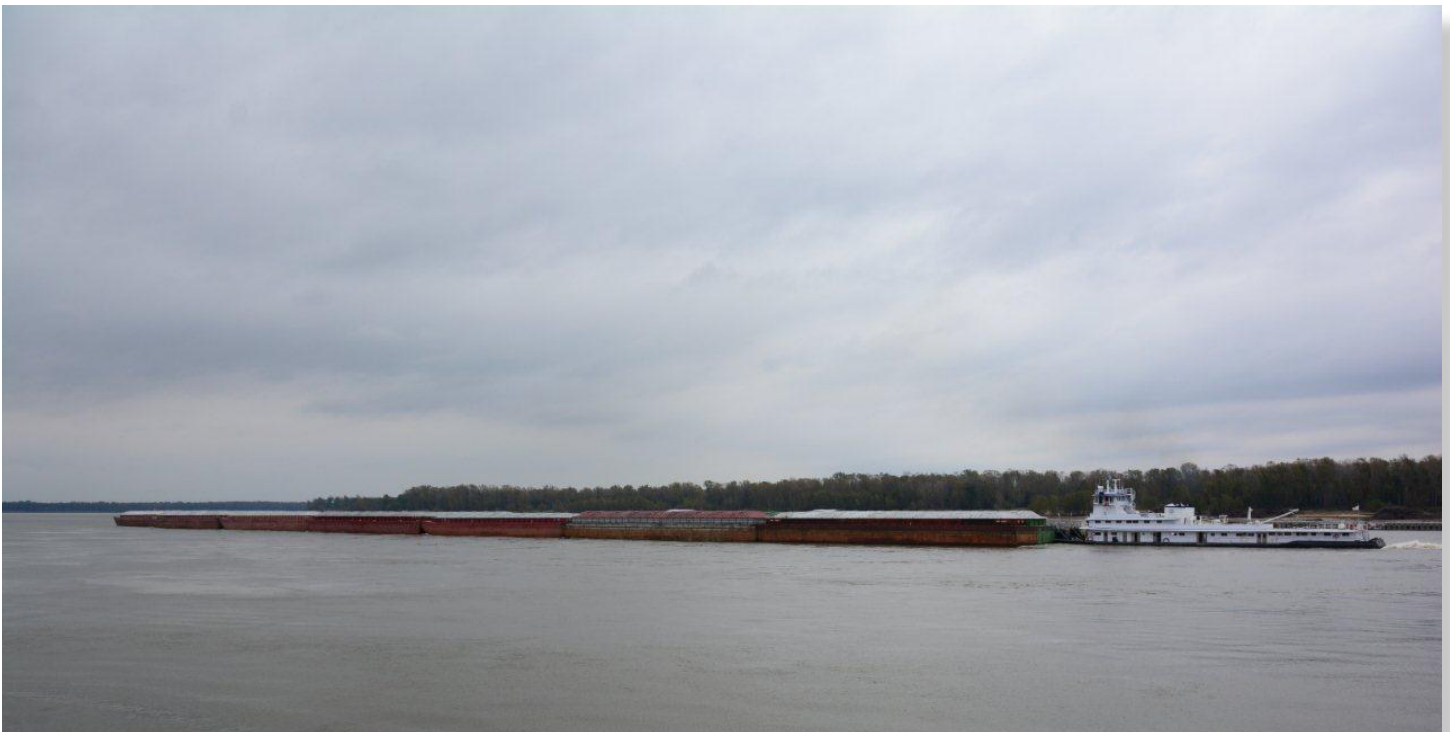
Revetment Work at Fair Landing, Arkansas —U.S. Army Corps of Engineers' Motor Vessel GRUGETT moves buoys on the Mississippi River to widen the navigation channel in order to minimize impacts to commercial navigation as revetment work progresses at Fair Landing, Arkansas, Nov. 9, 2014. The video of this work can be viewed at https://www.youtube.com/watch?v=3mVtkw9ZOGs&list=UUUp3ZXBw6xCuKExo4uBOjotQ . (Mat sinking unit photo courtesy of the U.S. Corps of Engineers.)
