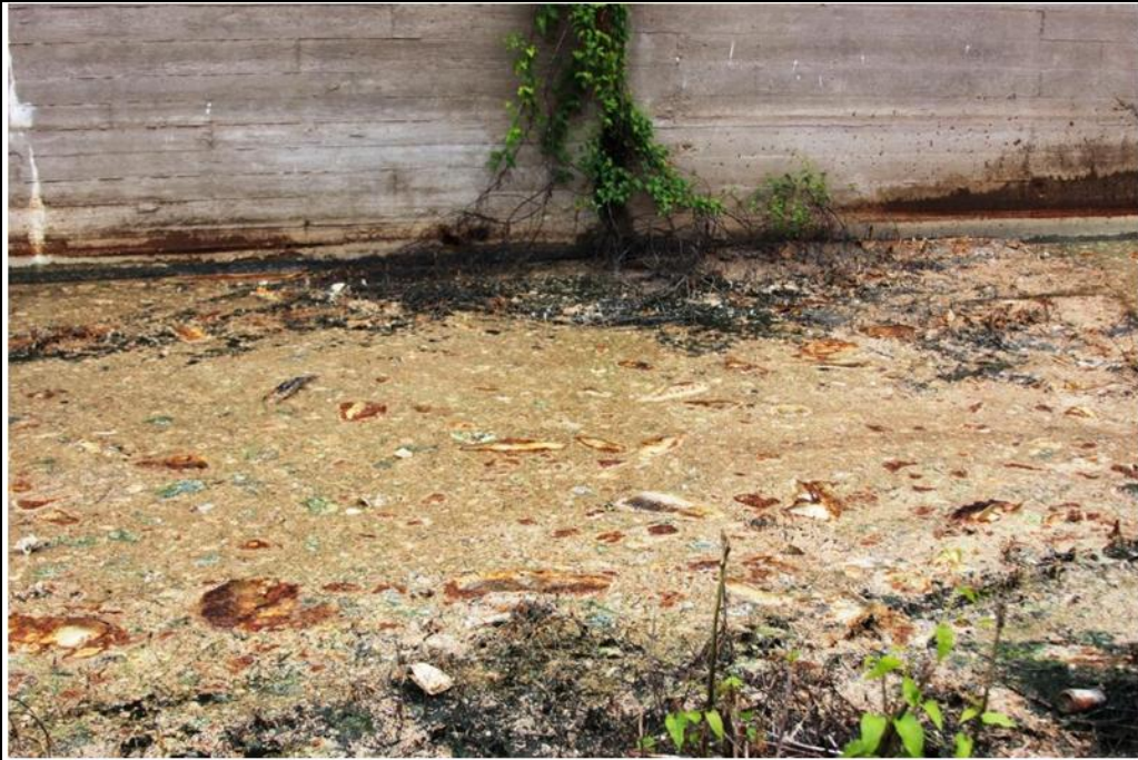
Figure 2.4. Rotten dead carp and buffalo below the Morganza Spillway structure.
