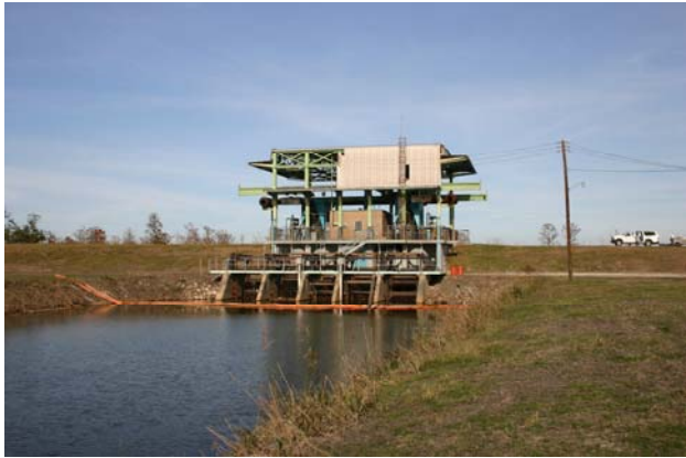
Figure 4. Station Sed 9 at Pump Station Meraux 4 on 40 Arpent Canal
