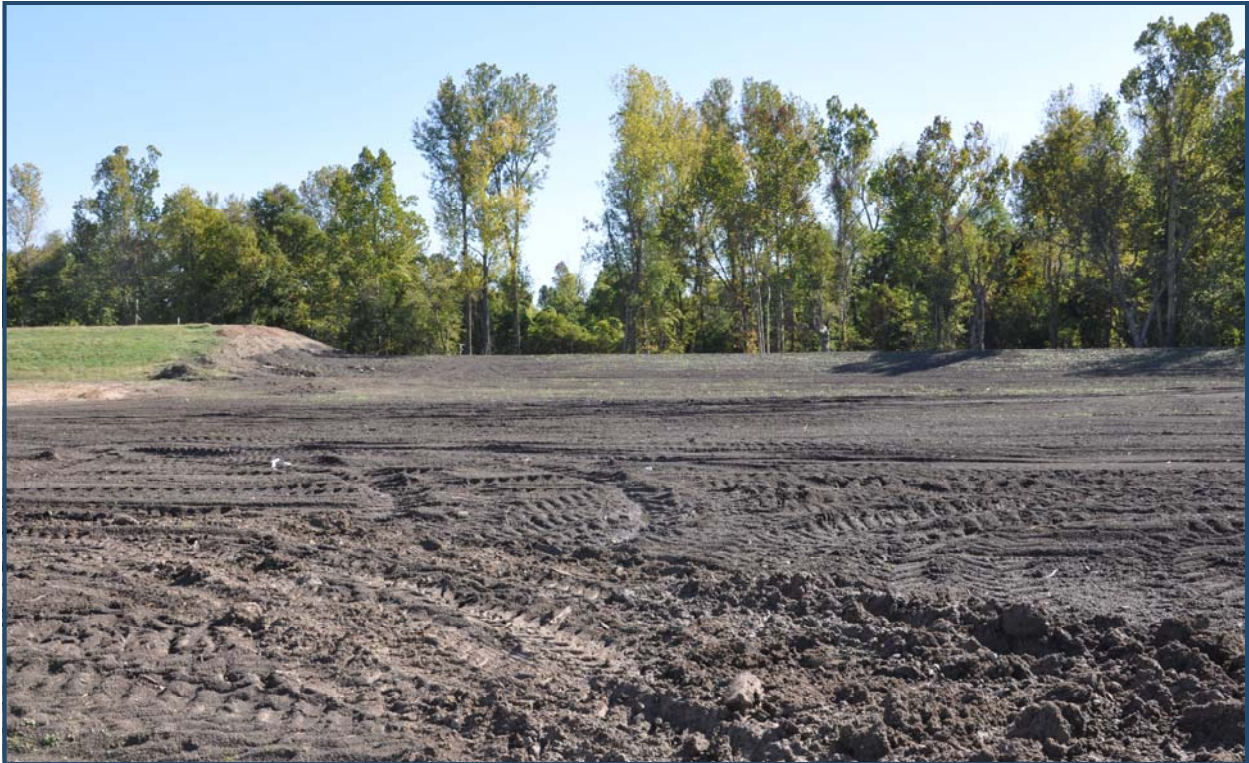
The extent of temporary repairs on the upper crevasse site at the Birds Point-New Madrid Floodway in late October 2012..
