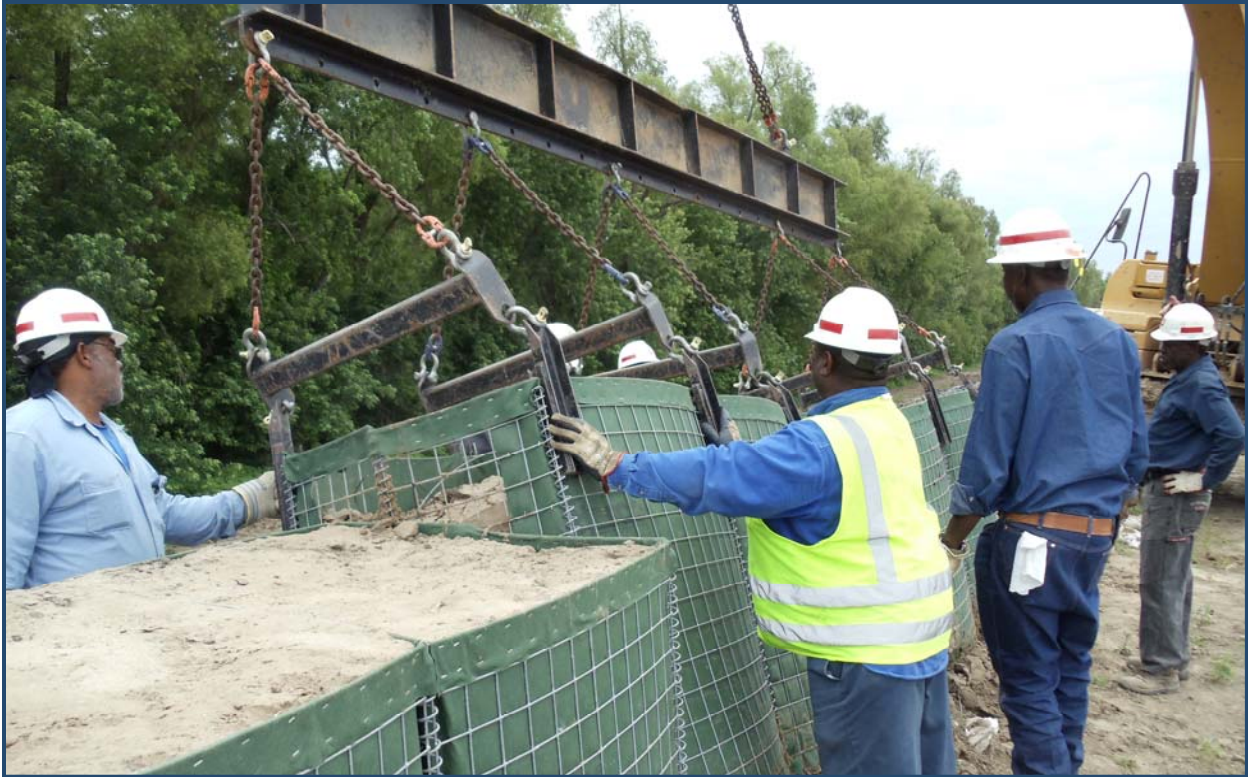
The extent of temporary repairs on the upper crevasse site at the Birds Point-New Madrid Floodway in late October 2012.
