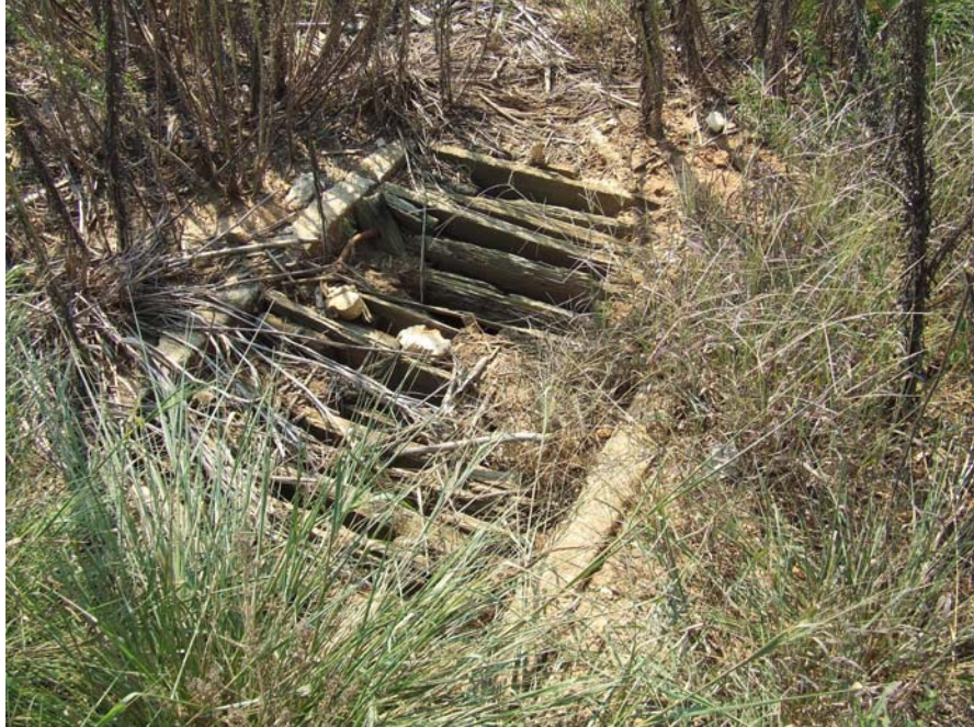
FIGURE 5 – Southeast View of Concrete Drain Associated With the 1942 Storm Water Drainage System (Photo by author)
