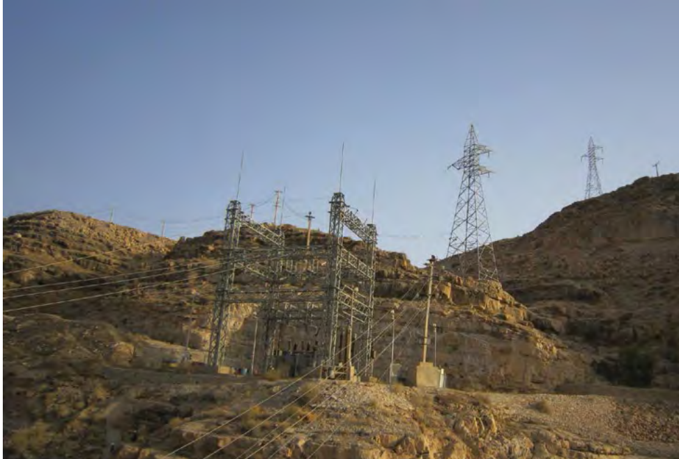
Insurgent attacks are also focused on non-military targets, including power transmission lines. (USACE photo)
