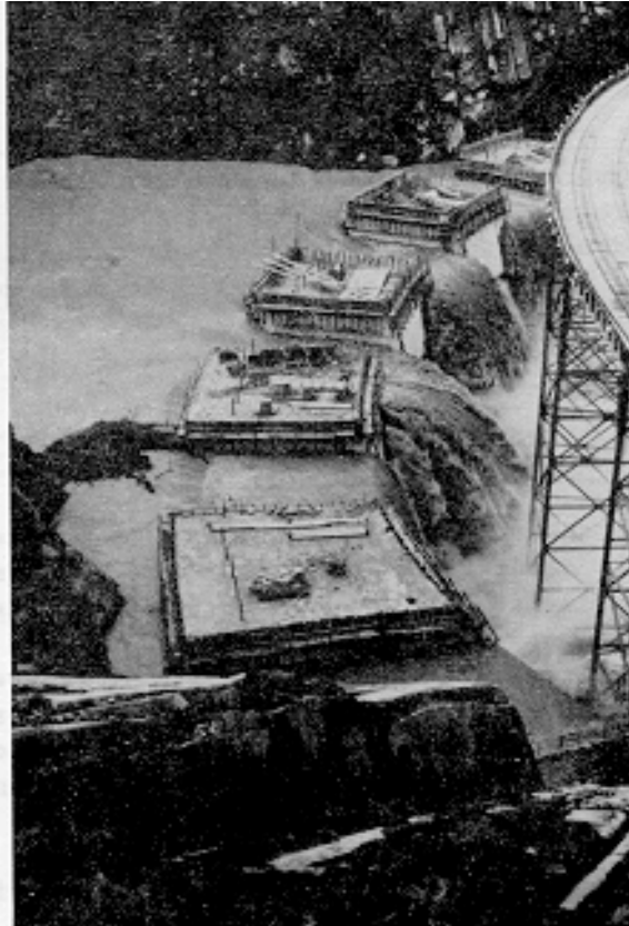
Figure 13-1. View from right abutment of partially complete Monticello Dam in California showing water flowing over low blocks (USBR)
