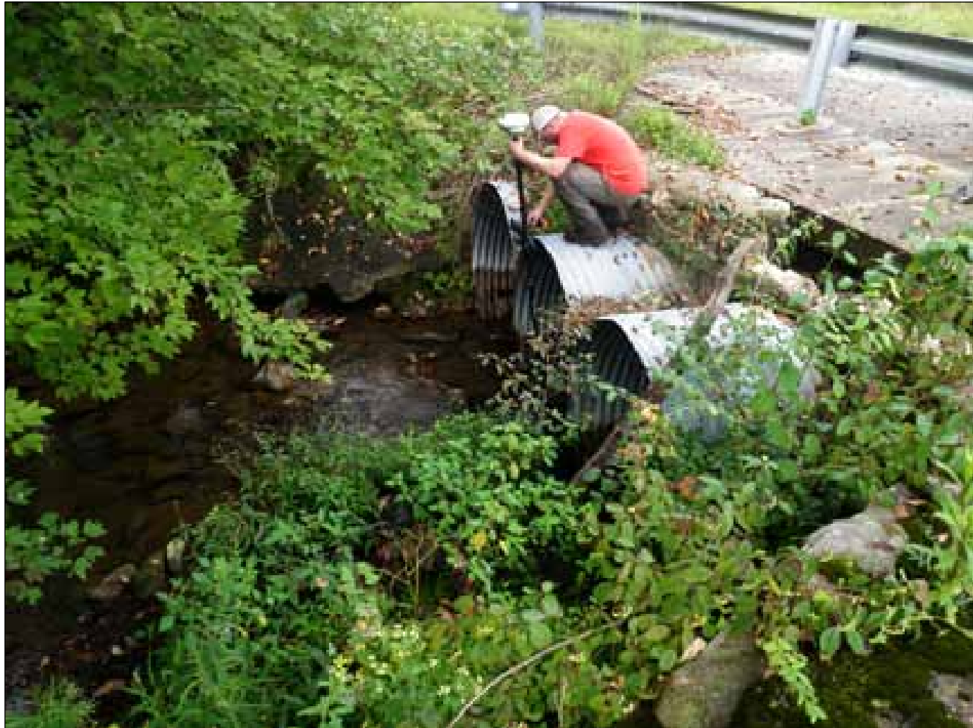
Baltimore District Geographer Karl Kerr uses the Real Time Kinematic survey equipment to gather the location and invert elevation of a culvert at Fort Indiantown Gap, Pa.. The data collected supported the development of the Chesapeake Bay TMDL. (Courtesy photo provided by the U.S. Army Corps of Engineers Baltimore District)
