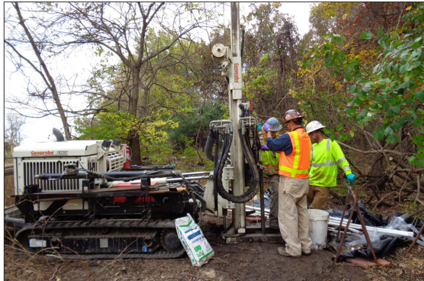
Contractors install sand lenses using direct-push technology and a custom injection system. (Courtesy photo)
