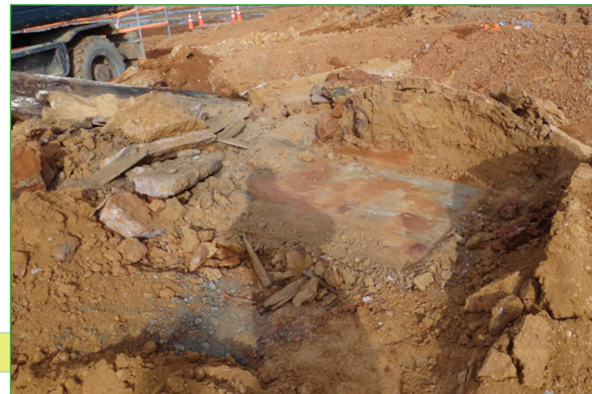
The Humphreys Environmental Division coordinated with the Republic of Korea Ministry of National Defense through U.S. Forces - Korea to properly relocate 11 grave sites that were discovered during excavation, while preparing for construction projects on the newly granted land. (Courtesy photo)
