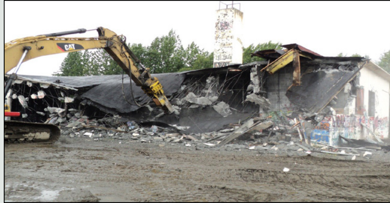
During the summers of 2010 and 2011, the Kenaitze Indian Tribe work crew demolished Wildwood Air Force Station's Buildings 100 and 101. The project was made possible by the Native American Lands Environmental Mitigation Program and conducted through a cooperative agreement with the U.S. Army Corps of Engineers Alaska District. (Courtesy Photo)
