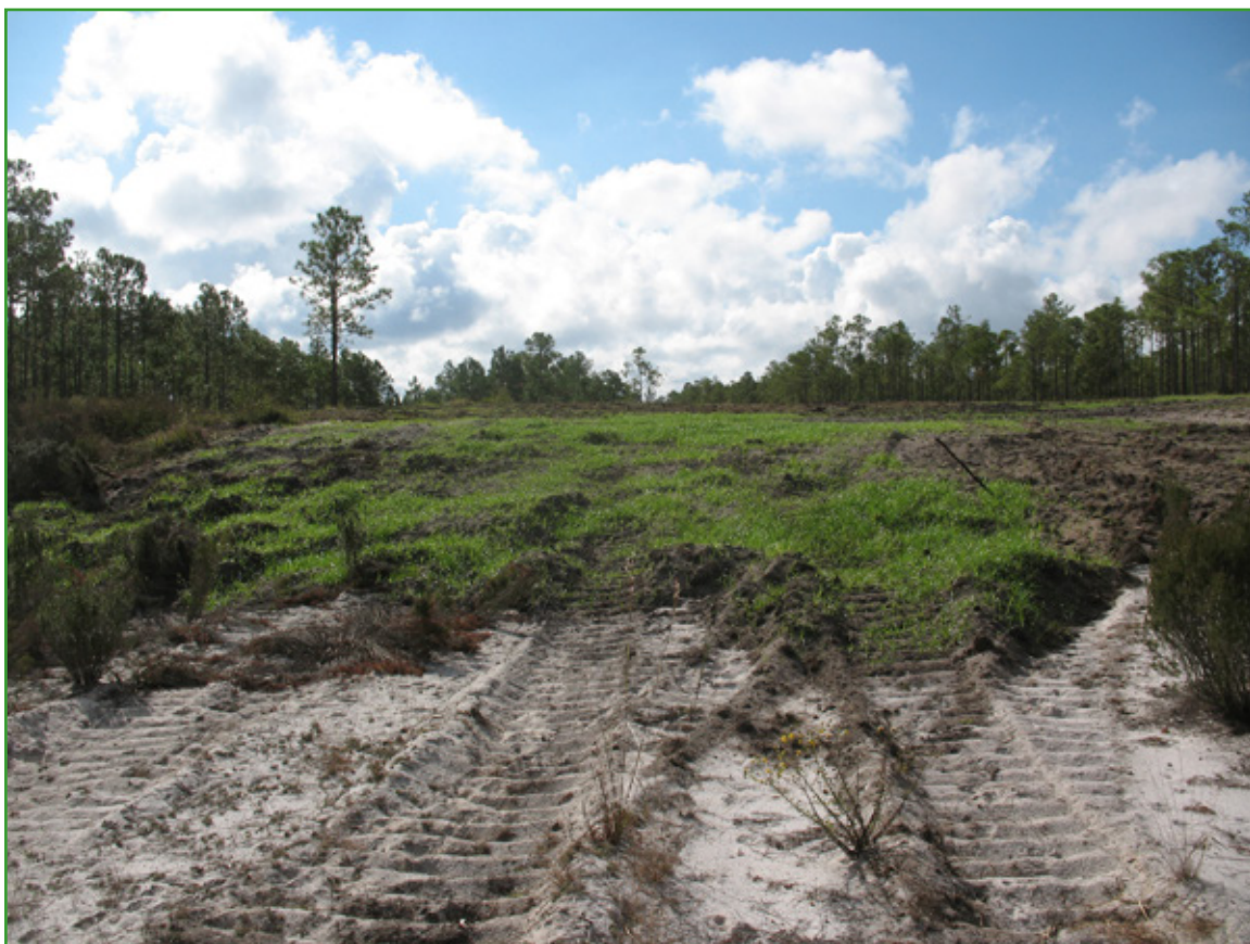
Vegetation sprouting in the project footprint contrasts with sparse wildflowers struggling in the sand beyond the current forward extent. The project is well on track to achieving its dual goals: remediation of the watershed landscape to prevent swale dirt from entering the river and establishment of a Florida-type ecosystem on the former mine sites that support vegetation and fire management. Last year, the first round of new tree plantings was completed at the mine site and, based upon early surveys, they are thriving with a remarkable survival rate of around 80 percent. (Courtesy photo)
