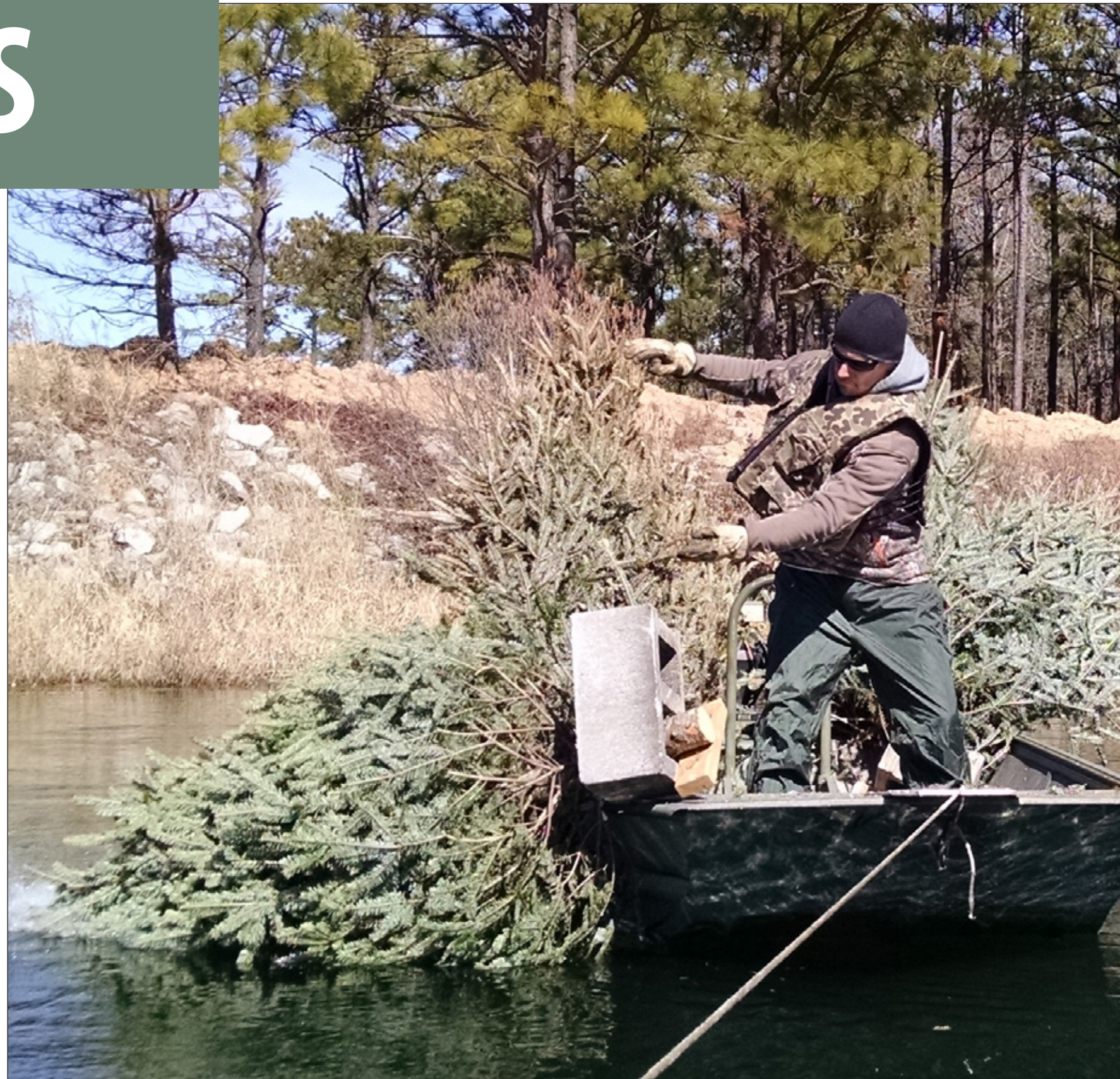
Travis Dodson, a wildlife technician with the Directorate of Public Works' Wildlife Branch at Fort Jackson, South Carolina, installs a fish attractor at Weston Lake. Twelve fish attractors were constructed using Christmas trees collected for recycling. The trees were anchored to the lake bottom by concrete blocks. "The structures will provide benefits to the aquatic community of the lake as well as to recreational fishermen," Dodson said. The branches of the submerged trees will immediately provide escape cover for small bait fish. Over time, algae and aquatic insects will colonize the trees, continuing to attract bait fish by providing them a food source in addition to cover from predators. As the bait fish congregate around the structure, larger predatory fish such as bluegill and largemouth bass will be attracted by the abundance of prey. Read more at www.army.mil/article/143528/ . (Photo courtesy Fort Jackson DPW)
