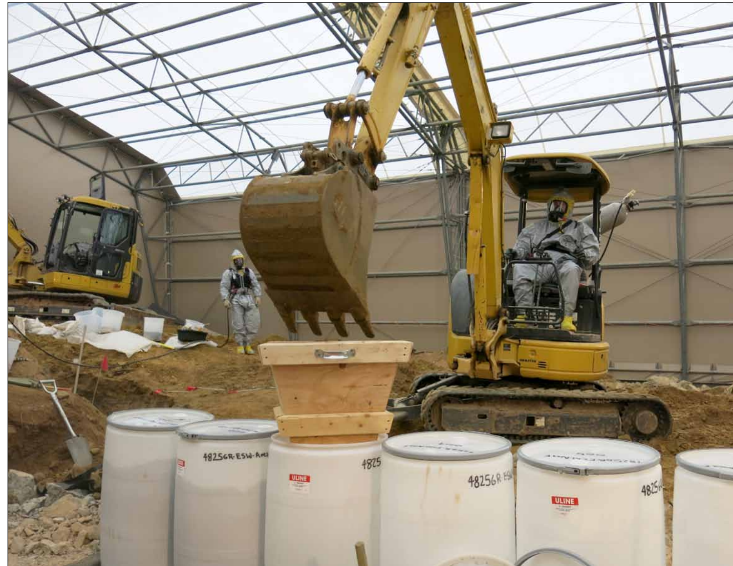
Crews continue excavations under high probability operations at 4825 Glenbrook Road, part of the Spring Valley formerly used defense site in Washington, D.C. (Photo courtesy Baltimore District)
