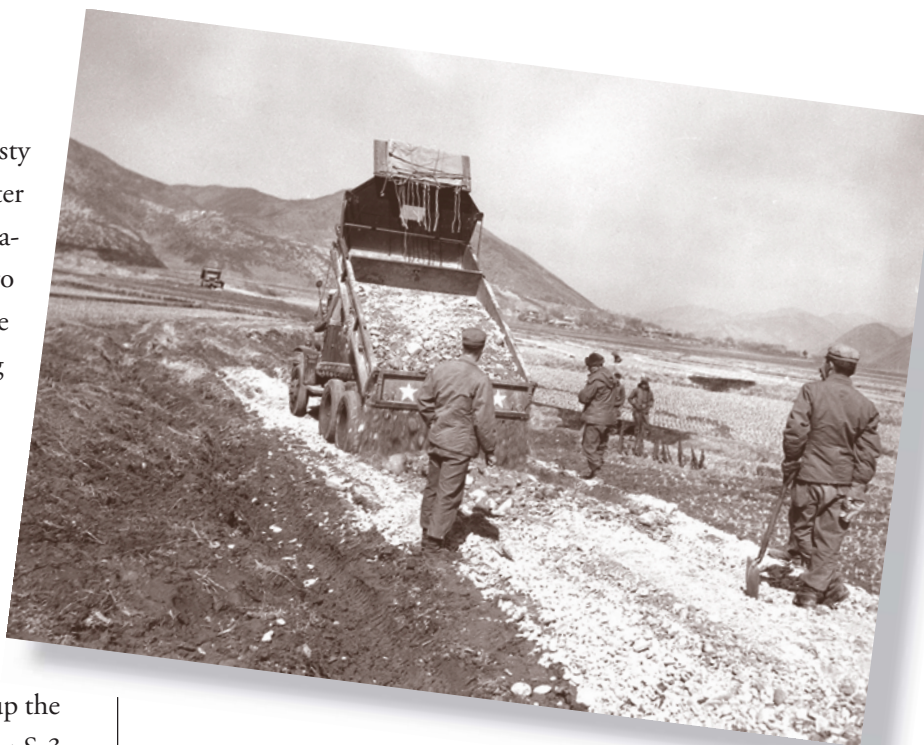
Men of the 65th Engineer Combat Battalion reinforce a muddy road on the north bank of the Han River Engineer School, 93-63-12
