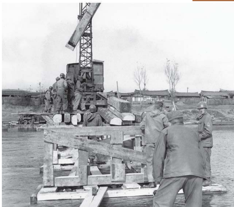
Soldiers of the 2d Engineer Battalion construct a timber trestle bridge across the Taedong River at Suncheon, 12 November 1950 Engineer School, 42-1-283
