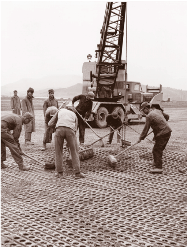
Engineers and Korean laborers repair a runway covered with pierced-steel planking Engineer School, 12-30-10
