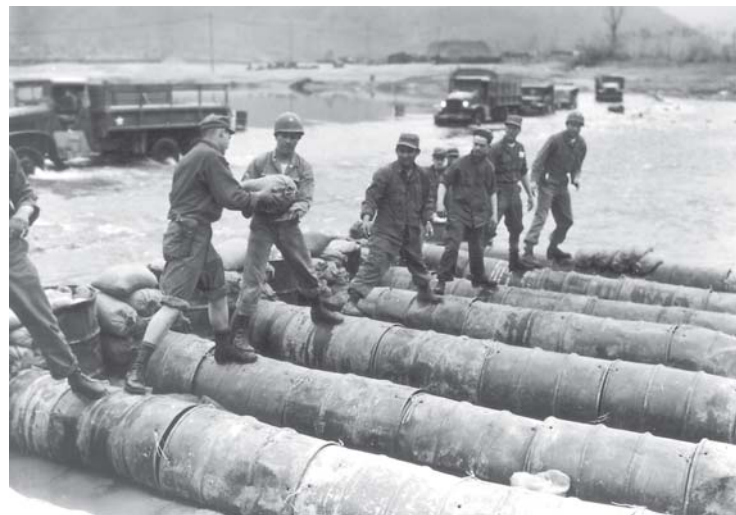
Using 55-gallon drums as culverts, the 378th Engineers construct a bridge over the Pukhan River RG 111, SC-364793
