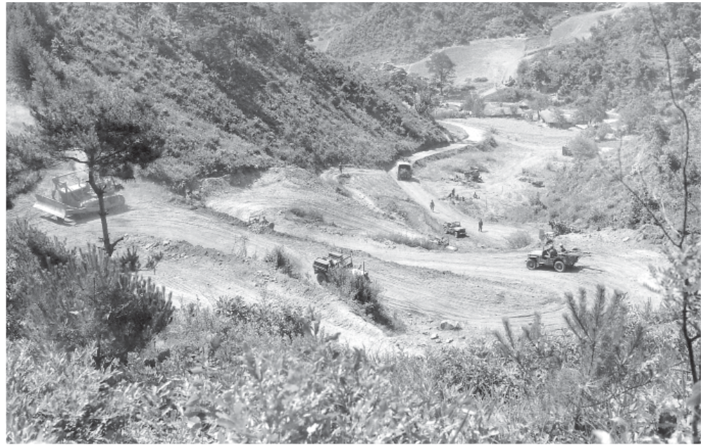
A road built by the 8th Engineers shows the hairpin turns needed to climb many of Korea's steep hillsides RG 111, SC-374167
