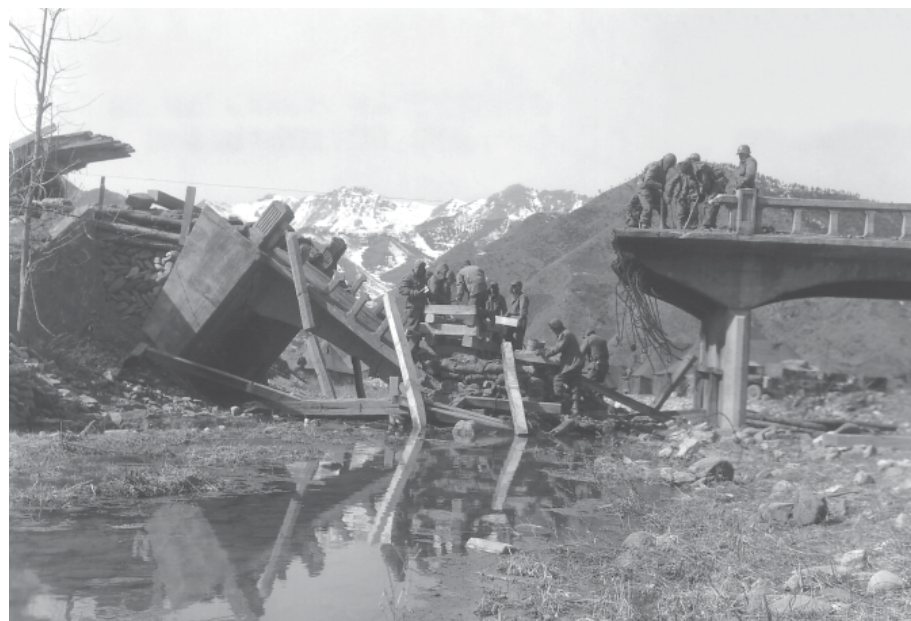
Soldiers of the 13th Combat Engineer Battalion repair a bridge destroyed by U.S. air power RG 111, SC-359632
