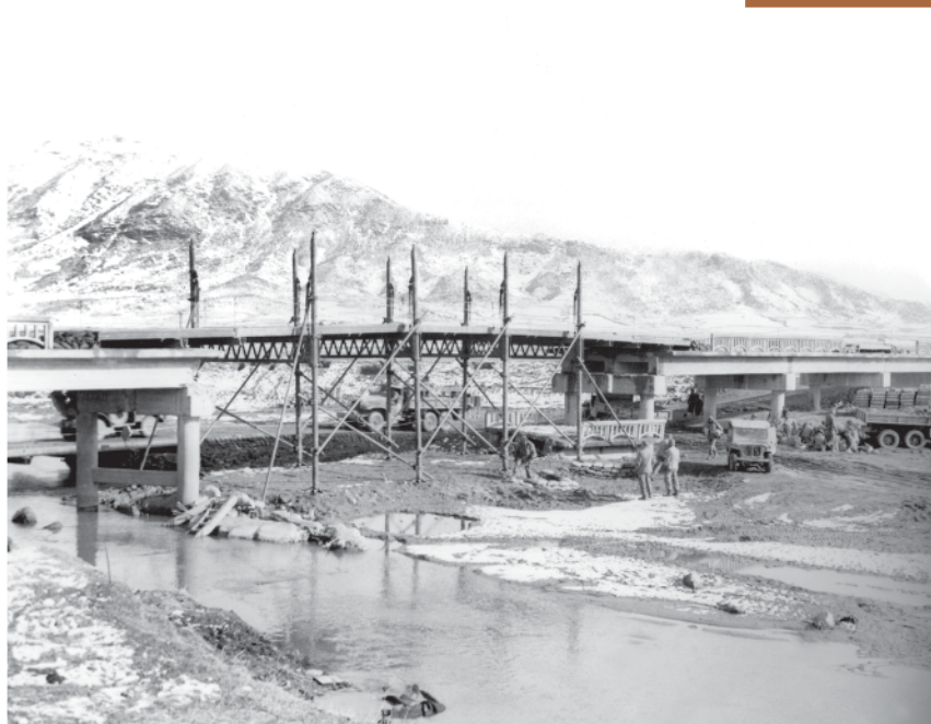
A fixed-trestle bridge built by the 10th Engineer Combat Battalion across the Han River Engineer School, Korea 084
