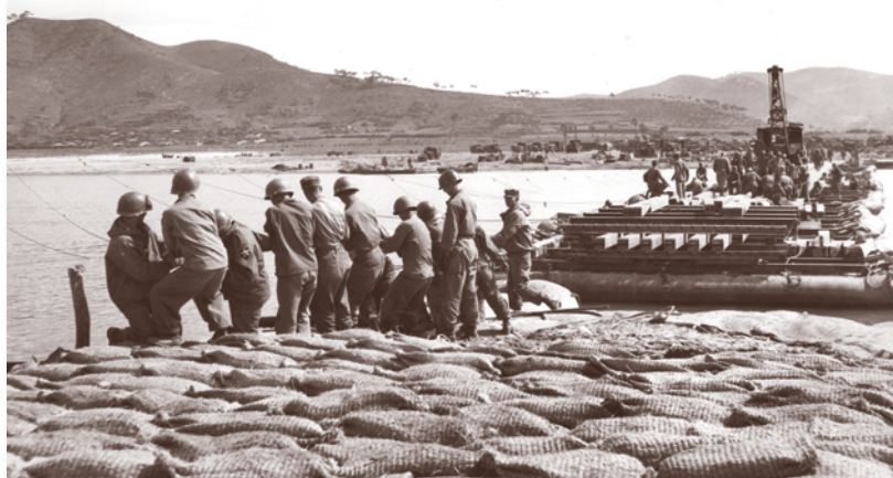
Engineers pull the last section of an M-4 ponton bridge in place over the Naktong River, 22 September 1950 Engineer School, 42-5-100
