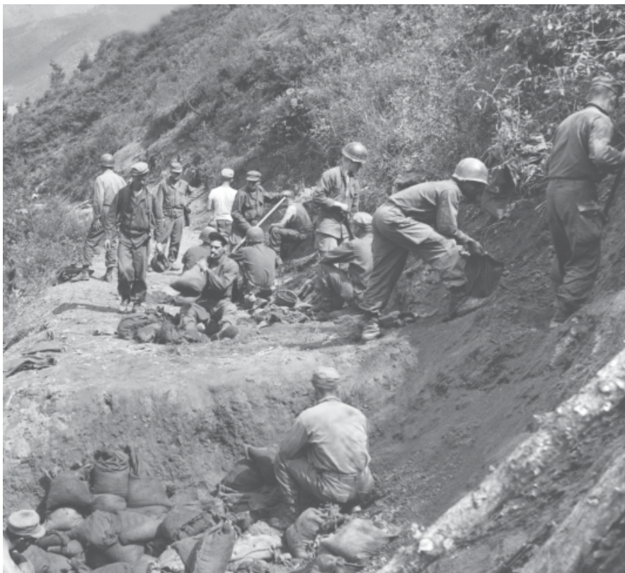
Men of the 13th Engineer Combat Battalion repair a road damaged by an enemy mine near Changp'yong, June 1951 RG 111, SC-369972
