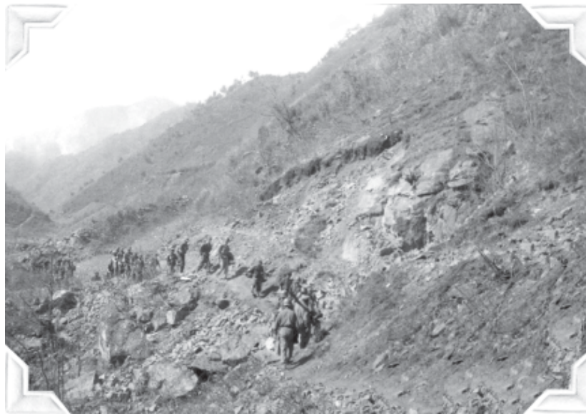
With the smoke of exploding artillery visible in the distance, infantry advance over a road cut by the 2d Engineers Love Collection
