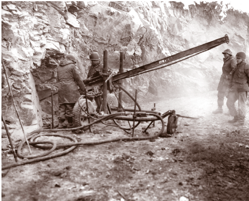
Soldiers of the 3d Engineer Combat Battalion use a wagon drill in preparation for blasting a hillside Engineer School, 71-11-23
