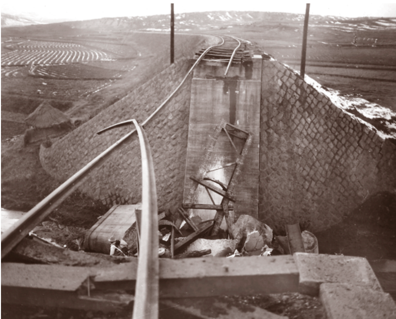
Engineers use 120 pounds of explosives, placed on the top of the pier and the inside of each beam, to destroy this railroad bridge RG 111, SC-359427
