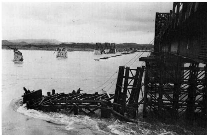
Figure 13. Pier from the collapsed high-level Teal bridge lodged against protective fender piles at the reopened span of the Freedom Gate bridge on 30 July 1952.
