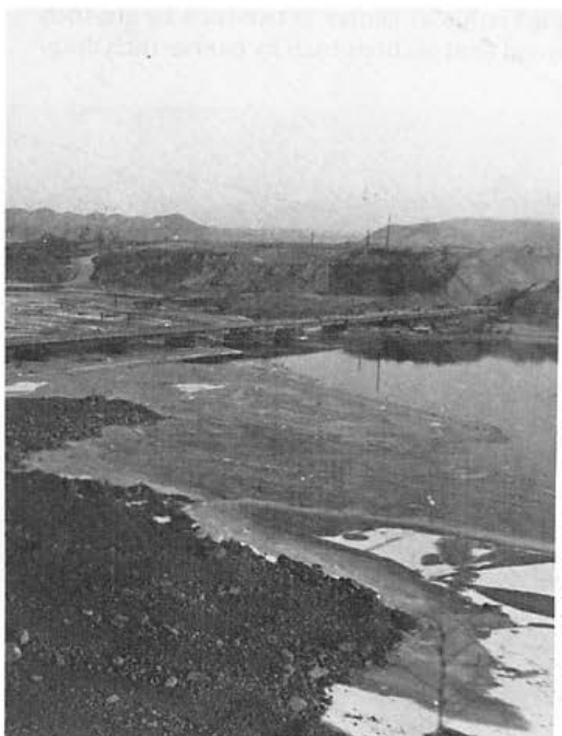
Figure 31. Teal bridge from the south shore on 7 January 1953 as troops place decking on the north end.
