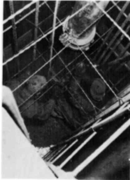
Figure 72. Inside pier 2 during D pour showing the pumpcrete pipe at top and the base for the pneumatic vibrator, used to assure proper placement of cement, at right.
