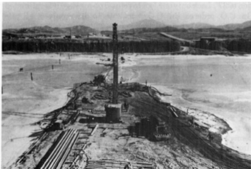
Figure 65. Excavation of cofferdam 6, begun by a 3\frac{1}{4} -yard clam bucket on 16 January 1953. Shower unit at lower left provided hot water for cement. Twelve inches of ice on the Imjin provided access to the far shore on foot.
