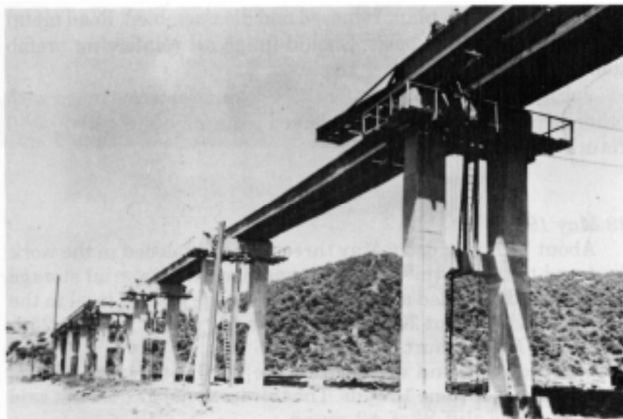
Figure 77. View showing portions of the 606-foot girders that were launched from the east abutment to pier 5. These were the longest girders used on the bridge.
