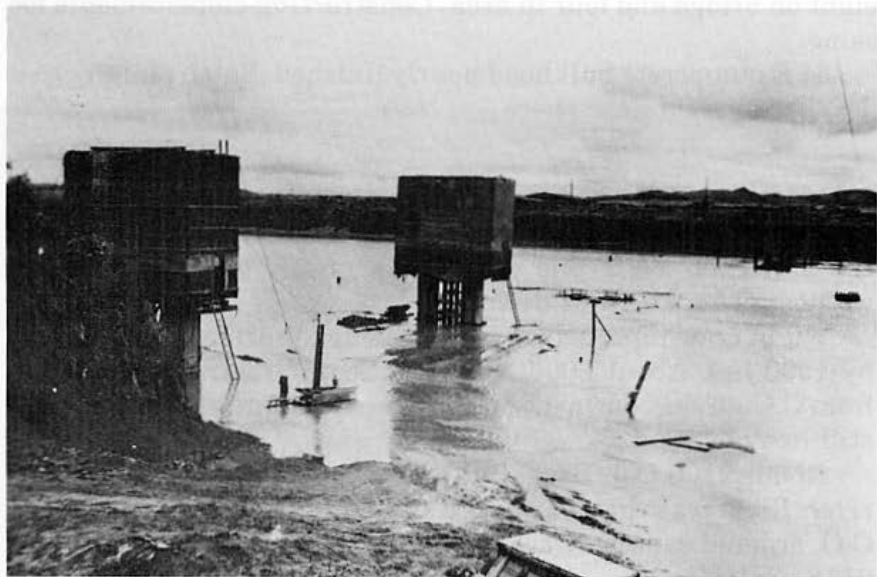
Figure 67. Storm water and a spring high tide combined to force an evacuation of the causeway on 20 March 1953. Piers 7 and 8 are in the foreground.
