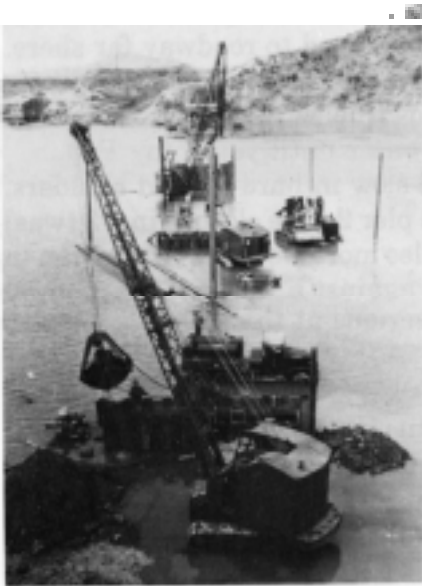
Figure 66. Work continuing on piers 1, 2, and 3 from submerged east causeway during high tide on 17 March 1953.
