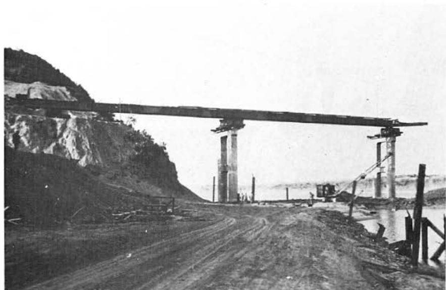
Figure 53. Steel beams in place from the west abutment across pier 8 to pier 7. The 30-foot launching nose may be seen beyond pier 7.
