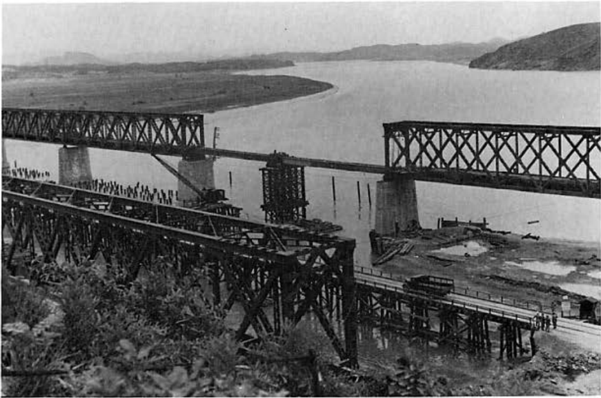
Figure 11. Construction under way to reopen the more southerly railroad bridge at the Freedom Gate site. The low-level pile bridge is visible at the right of this 9 July 1952 photo.
