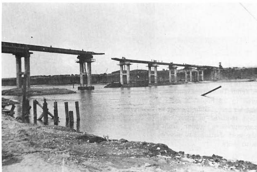
Figure 54. Launching the span across piers 7, 6, and 5. Launching noses extend both east and west into the gap between piers 5 and 6.
