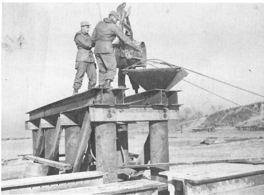
Figure 24. Troops filling the hollow Armco piles with concrete, with 36-inch I-beam girders in the foreground.
