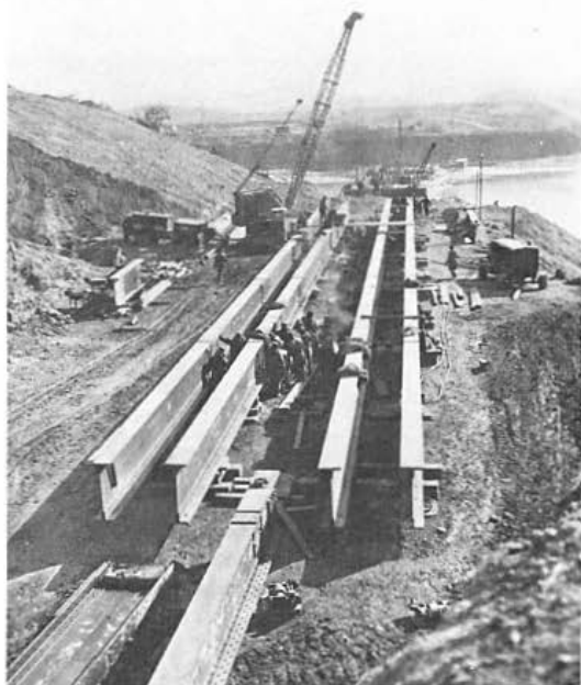
Figure 52. Steel beams being prepared for the span from the west abutment to pier 7, while riveters received training on the beam at left center.
