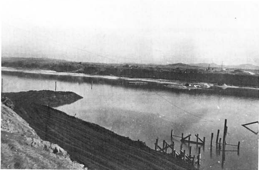
Figure 38. The Imjin River at the X-Ray site, showing early progress on the construction causeway and test piles driven in November 1952 to determine the depth of bedrock.
