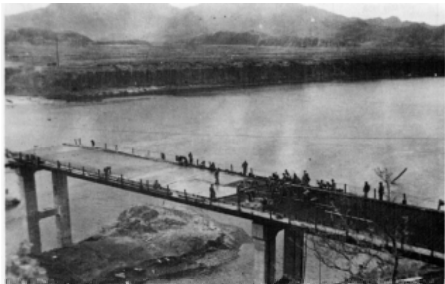
Figure 75. Troops laying the concrete deck. Two steel mats reinforced the concrete to provide an "antiartillery" safety factor beyond the necessary load-carrying strength. The concrete placing was monolithic and continuous.
