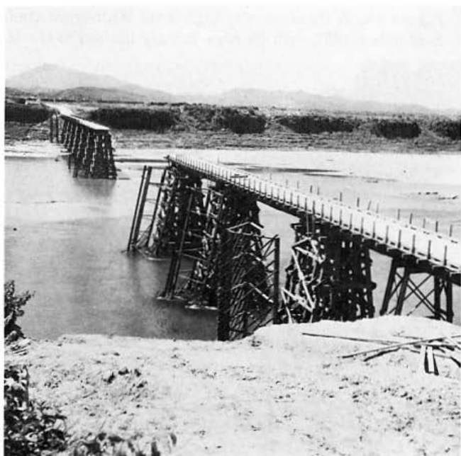
Figure 14. The high-level Teal bridge in early August 1952, showing damage done by floodwater on 30 July.
