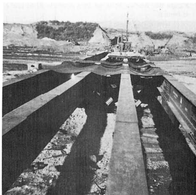
Figure 27. Thirty-six-inch I-beams in place on bridge with a pile driver, in background, working on one of the northernmost piers.
