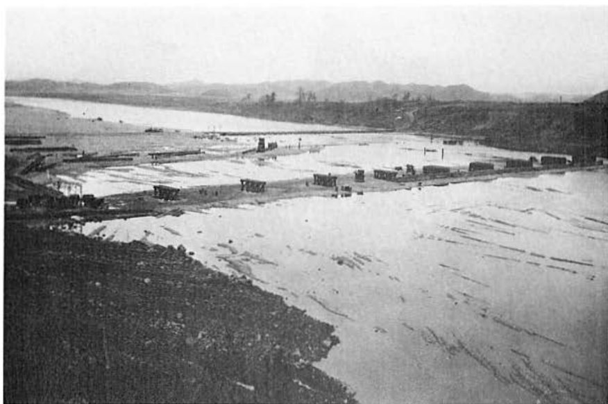
Figure 26. Teal site on 26 November 1952 showing completed piers at south end of bridge, left, and others still under shelters. I-beam girders and the Imjin River flowing north of the causeway are visible at right.
