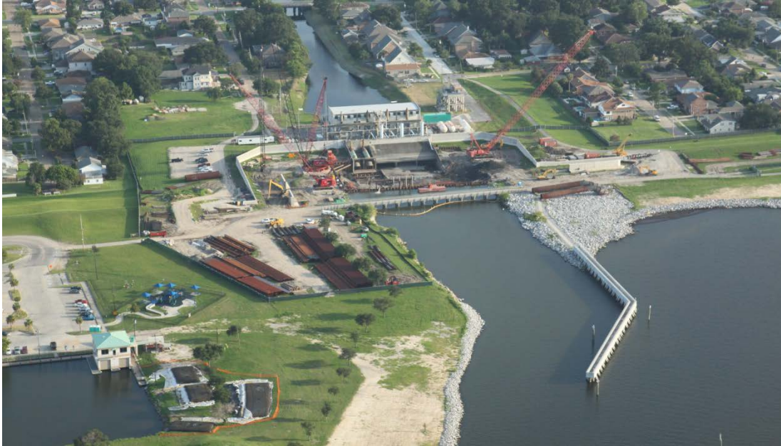
Aerial image taken in July 2012 of ongoing fronting protection construction at Bonnabel Pump Station.
