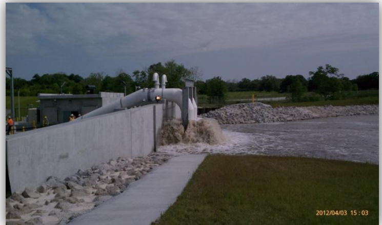
WBV-09a Pump station along Oakville Levee
