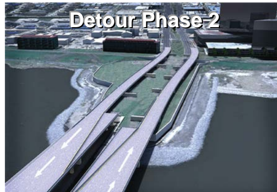
In the second phase of construction Causeway travel lanes were detoured onto the newly constructed elevated lanes.
