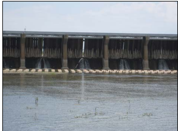
Photograph 5-1. Leakage through the spillway structure during high water events on the Mississippi River
