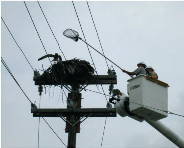
An installation conservation law enforcement officer gets assistance from NASO utilities crew and equipment to rescue a juvenile osprey from a nest located on a utility pole at NASO Dam Neck Annex that caught fire earlier in the day after a storm event.
