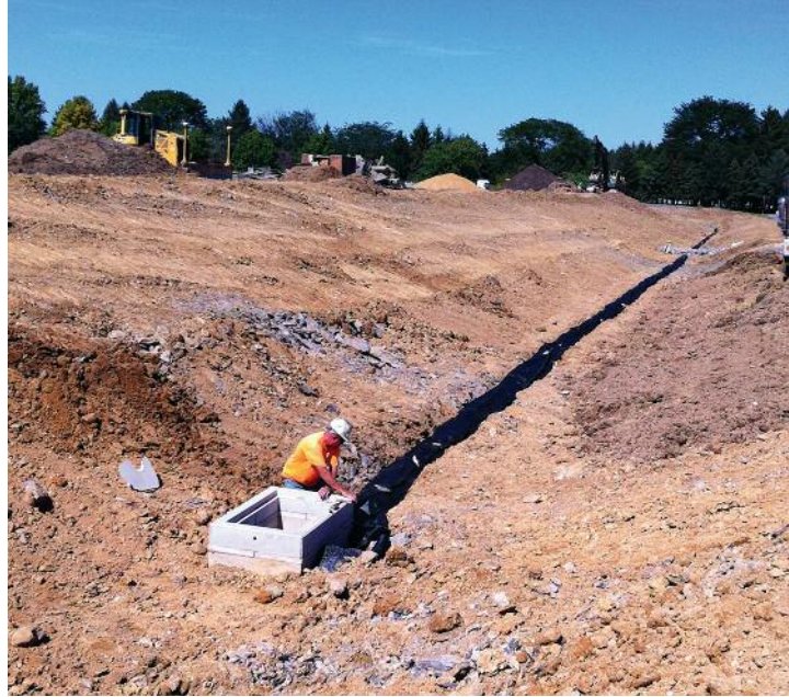
The excavation and bottom drain for a 600 by 200 foot bioretention area for reducing pollution in stormwater runoff. Best management practices implemented during the award period such as this one will reduce stormwater runoff of nitrogen, phosphorus, and suspended solids by over 11 tons per year.
