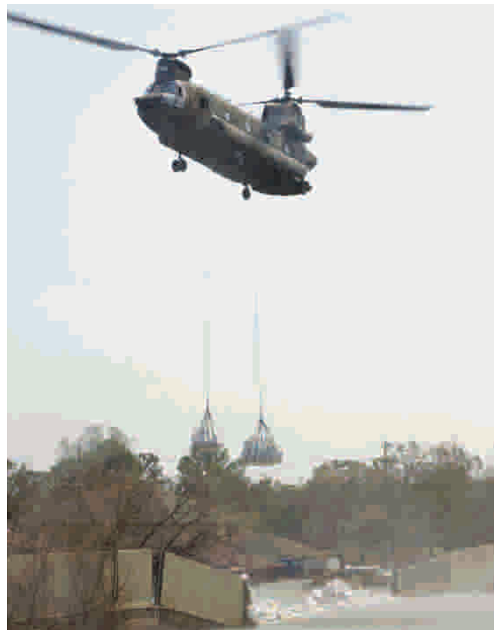
A CH-47 moves into position to drop a sling-load at the break in the 17th Street Canal, 10 September 2005. The 149th Aviation Support Battalion, Texas Army National Guard airlifted and strategically dropped bundles of rock and sand at the break in the 17th Street Canal, which collapsed when Hurricane Katrina hit New Orleans, Louisiana. U.S. Air Force photo by Master Sgt. Scott Reed.
