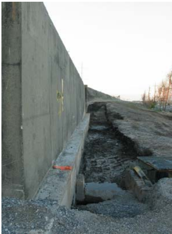
Figure 4.4. Scour trench at a T-wall on the east side of the IHNC
