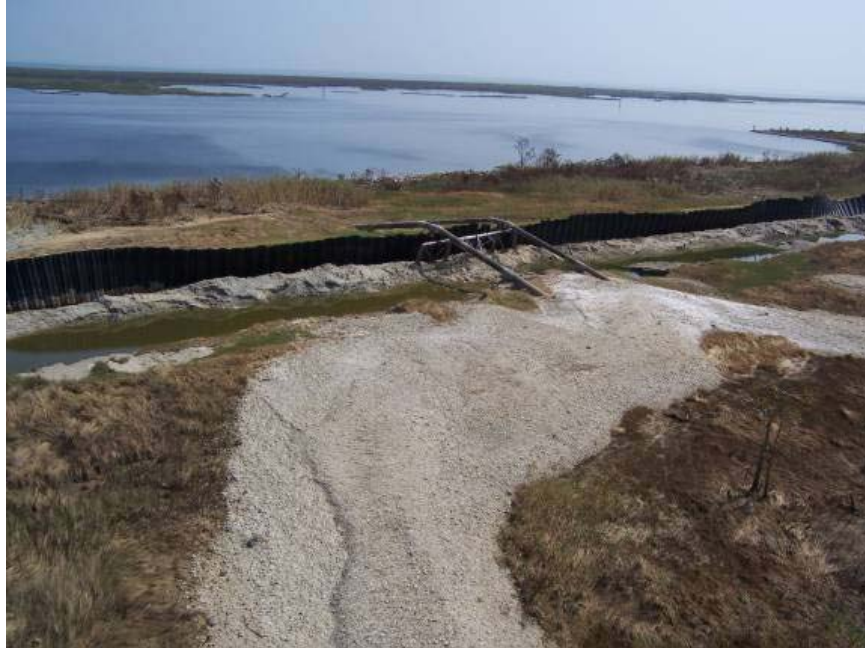
Figure 4.5. Overtopping scour at sheetpile floodwall along the MRGO
