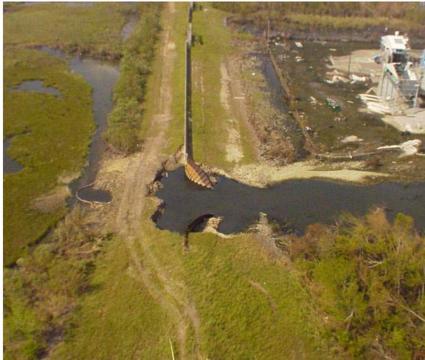
Figure 4.6. Sheetpile floodwall breach on the New Orleans East Back Levee
