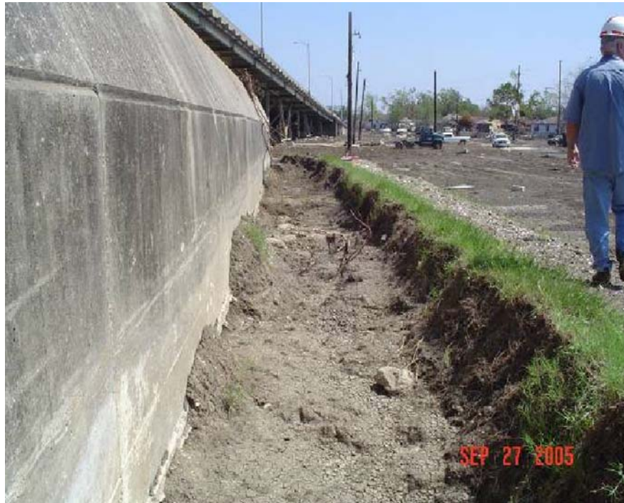
Figure 4.3. Scour trench on the east side of the IHNC
