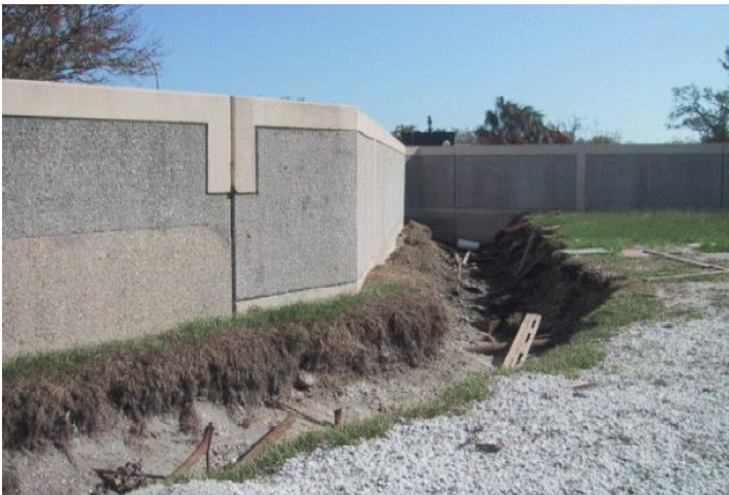
Figure 4.2. Scour trench formed by overtopping flow at I-wall adjacent to the Lakefront Airport (photograph by Peter Nicholson from Seed, et al. (2005)).
