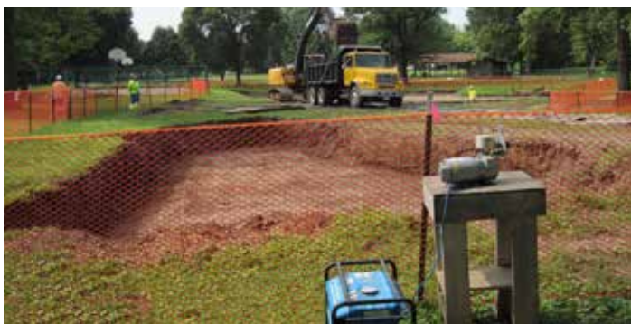
St. Louis Airport Site Vicinity Properties excavation at St. Cin. Park adjacent to Coldwater Creek
