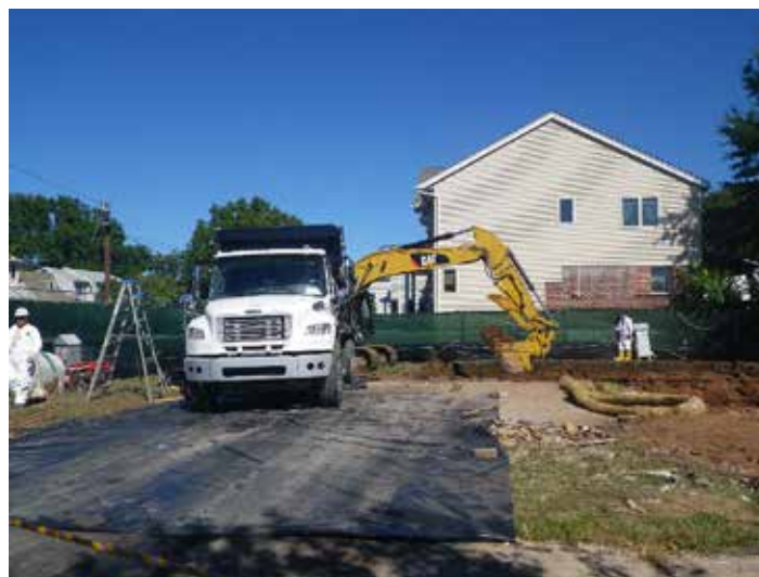
Remedial excavation begins at the site of a demolished home in Lodi, New Jersey. Demolition was the most cost-effective option to access contaminated soil beneath the home.
