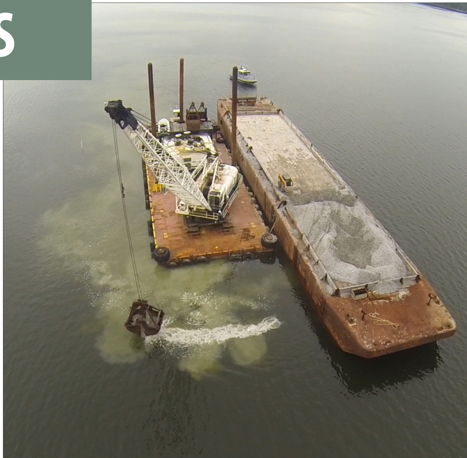
Contractors working for the Norfolk District U.S. Army Corps of Engineers place fossilized shell, obtained from the Virginia Marine Resources Commission, on sanctuary reefs in the Great Wicomico River in Burgess, Virginia, in July. The reefs, originally built by USACE in 2004, are receiving the new shell as part of an adaptive management/rehabilitation project, which is building them up to a higher level promoting a healthier oyster reef. (Photo by Patrick Bloodgood, Norfolk District)
