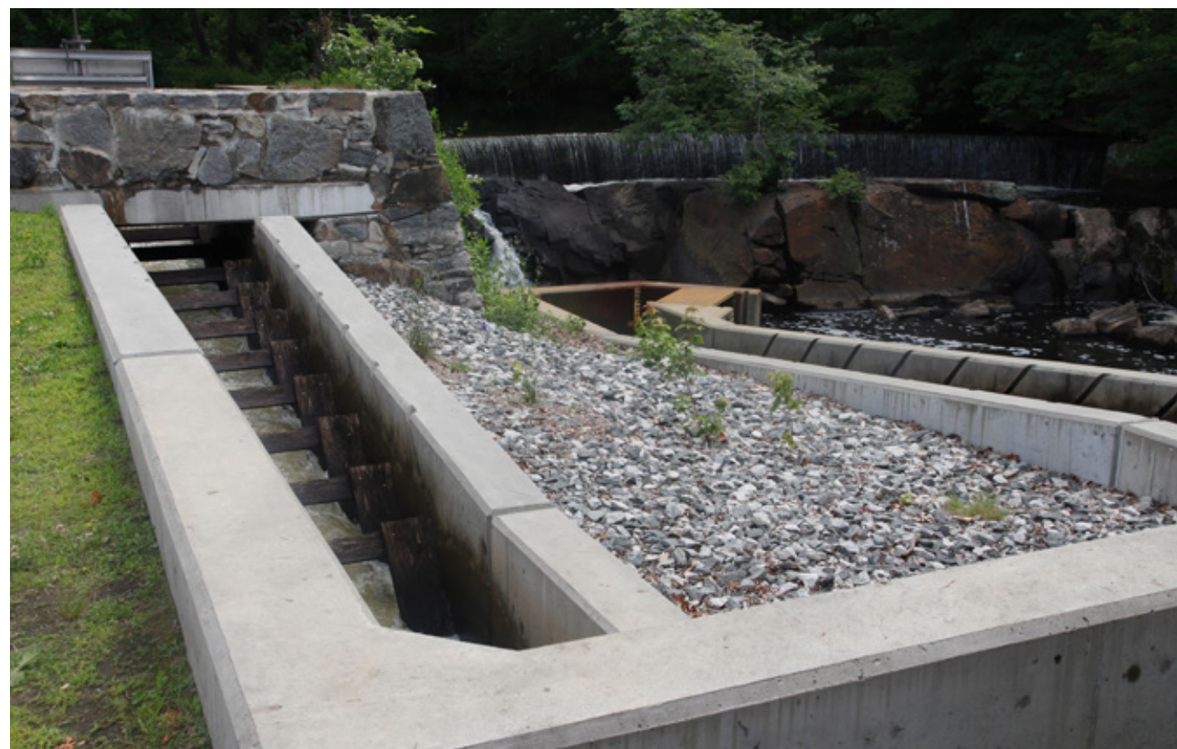
One of the fish ladders constructed along the Ten Mile River. The Denil Fishways provide for upstream migration of anadromous fish to their historic spawning areas (Photo by Brian Murphy)
