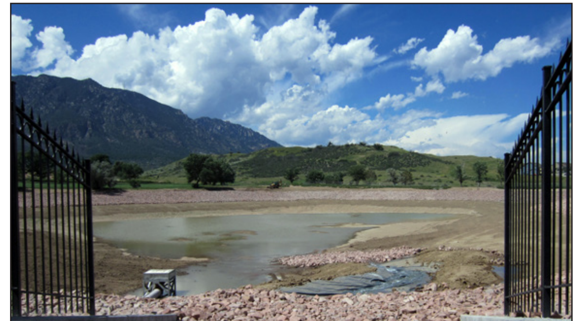
A large-scale project to expand the reclaimed water system to irrigate the majority of the turf areas on Fort Carson included expanding the Cheyenne Shadows Golf Course holding pond to hold up to 16 million gallons of water for use during watering season. (Fort Carson Directorate of Public Works)
