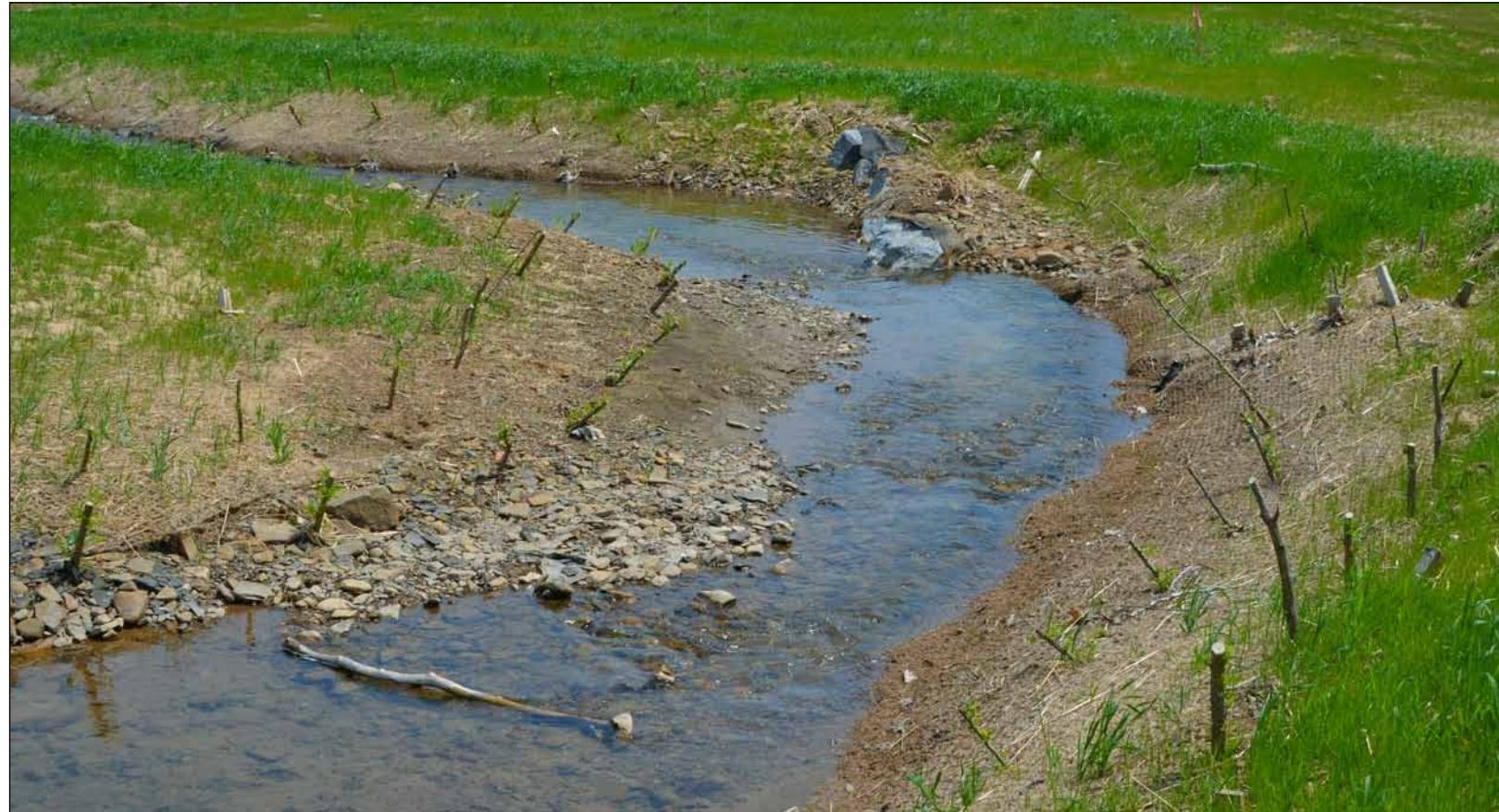
This stream is undergoing restoration at a mitigation bank site in Spanishburg, West Virginia. Mitigation banks, and other compensatory mitigation strategies, help make natural resources exploration, extraction, processing and other development activities possible, while protecting aquatic resources and their functions. (Courtesy photo)
