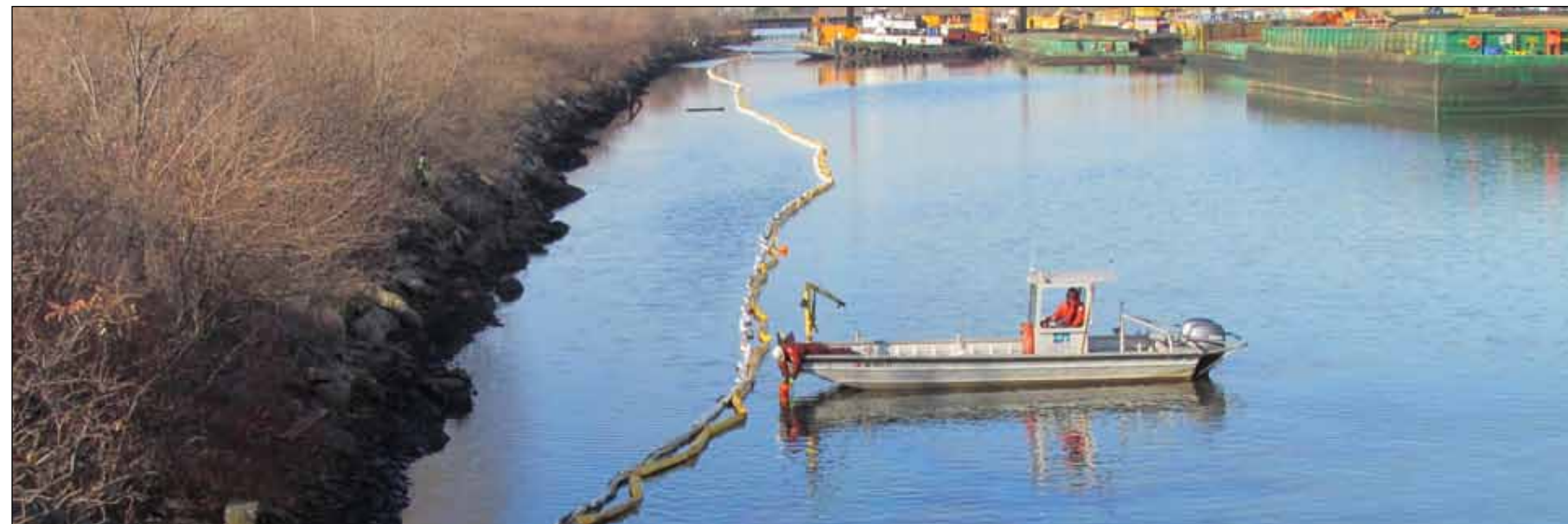
A worker installs oil booms at Indiana Harbor and Canal, Nov. 27. (Photo by Vanessa Villarreal)
