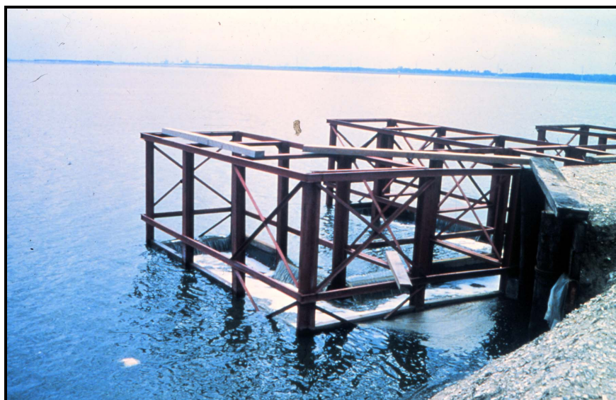
Figure 24. Conventional Weir with Boards
