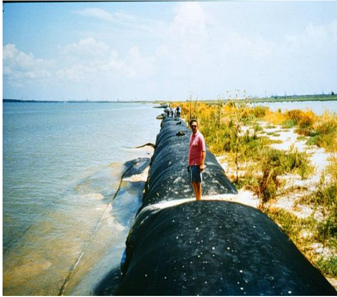
Figure 21. Geotube/Salt Marsh, Bayport, TX
