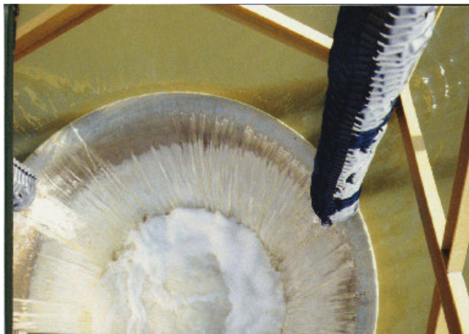
Figure 26. Effluent Flowing Over Telescoping Weir
