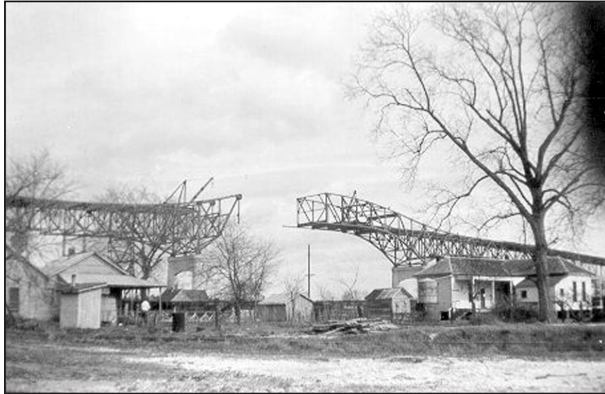
Figure 5-21. Construction of the superstructure of the new Calcasieu River Bridge in circa 1951 (Carpenter 2005) as viewed from Old Westlake.
