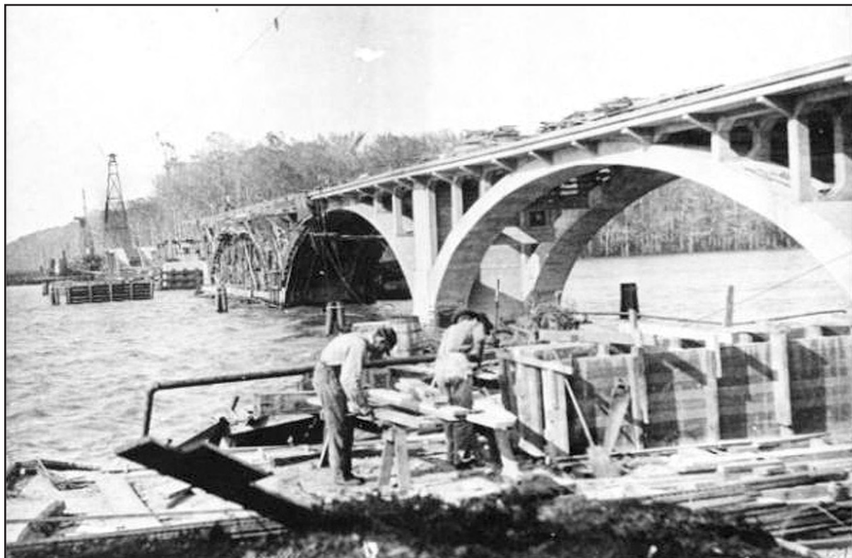
Figure 5-18. Construction of the first Calcasieu River bridge in circa 1915 (MSU Photograph No. 112, Frazar Memorial Library, McNeese State University, Lake Charles, Louisiana). The bascule bridge served as an integral part of the Old Spanish Trail and later as part of U.S. 90 until it was demolished in June 1953.
