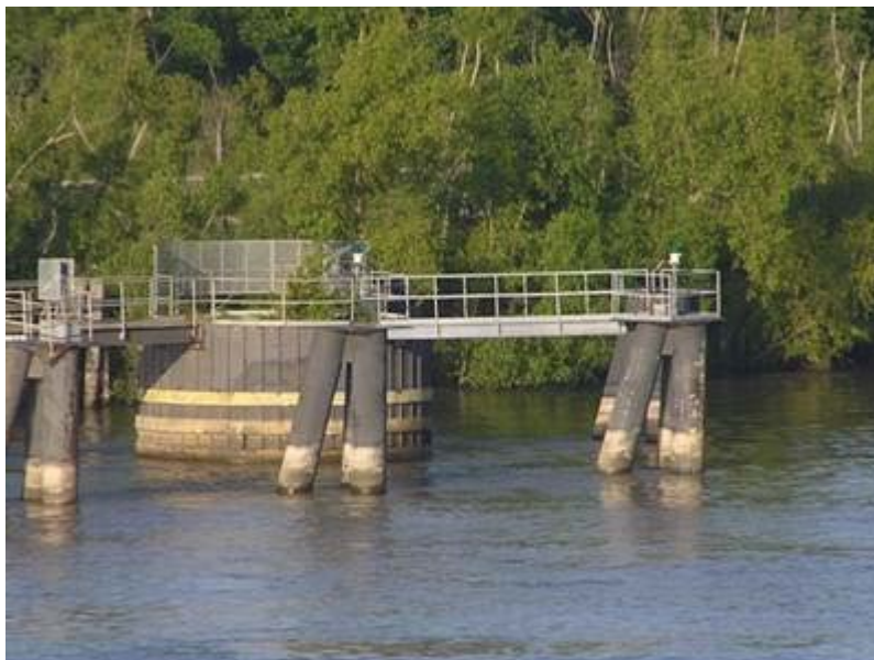
Mooring dolphins fabricated from steel pipe piles
