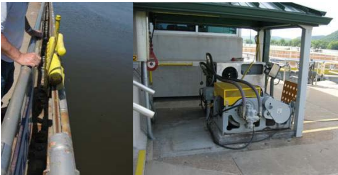
A rail-mounted travelling kevel unit and powered winch system (Photos courtesy St. Paul District)
