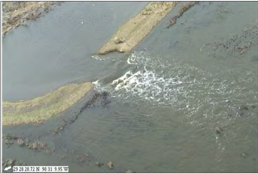
Figure 2-3. Breach at West Corner of “Stair-Step” Portion of Montegut Non-Federal Levee
