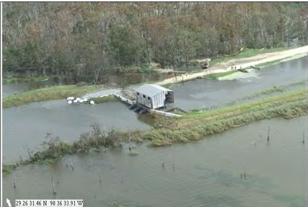
Figure 2-4. Breach at Lashbrook Pump Station on Ward 7 Levee along Boudreaux Canal Scour has undermined timber fronting protection, allowing water to seep under pump station.
