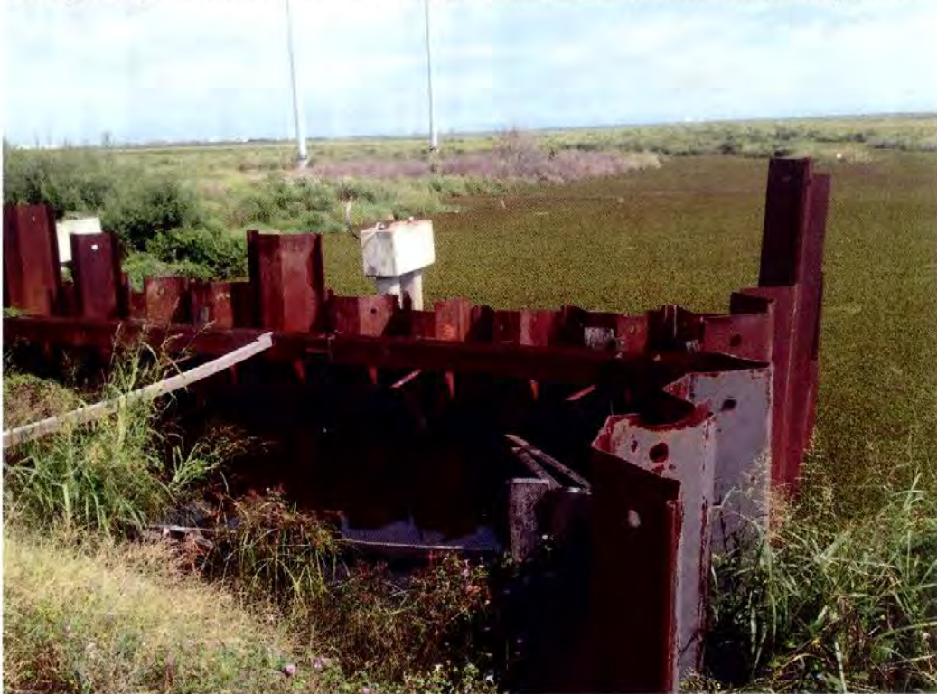
Photograph 2. St. Bernard Parish Pump Station #3 flood side wetland edge vegetation and existing sheetpile cofferdam. Invasive duckweed covers almost the entire discharge basin.
