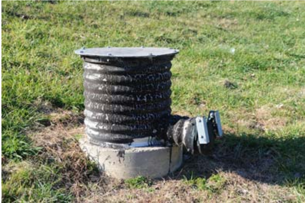
Figure 2: Typical Relief Well - The typical relief well has a diameter of 8 inches and stands approximately 20 inches above ground. A concrete pad may or may not be present to direct flow from the well.
