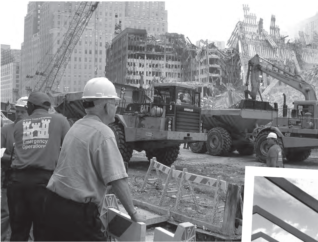
Above: The Corps of Engineers responded to the terrorist attacks of September 11 at the Pentagon and in New York.
