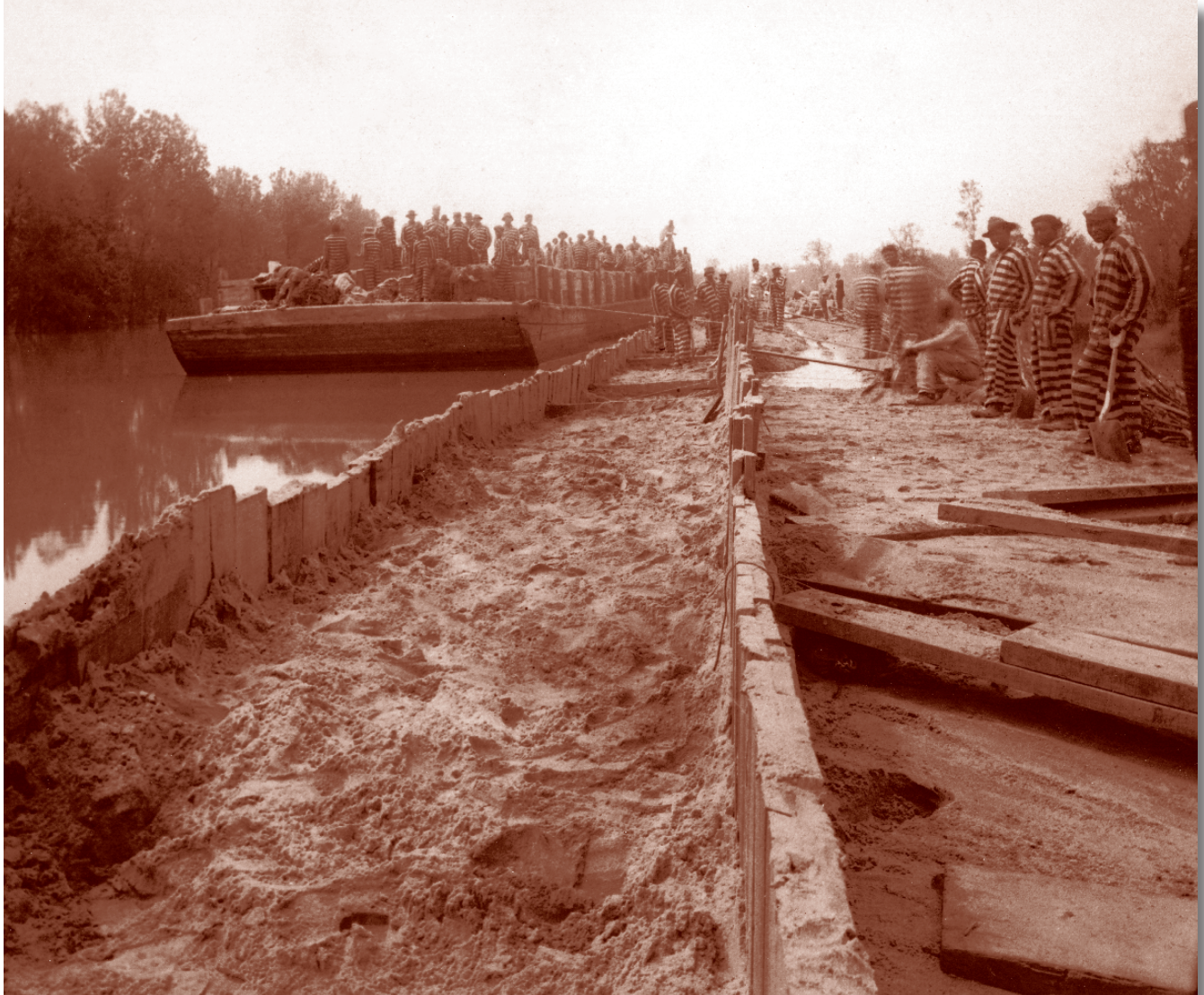
Convicts constructed a mudbox atop a levee near Fulton to hold out the Mississippi River flood in 1927.
