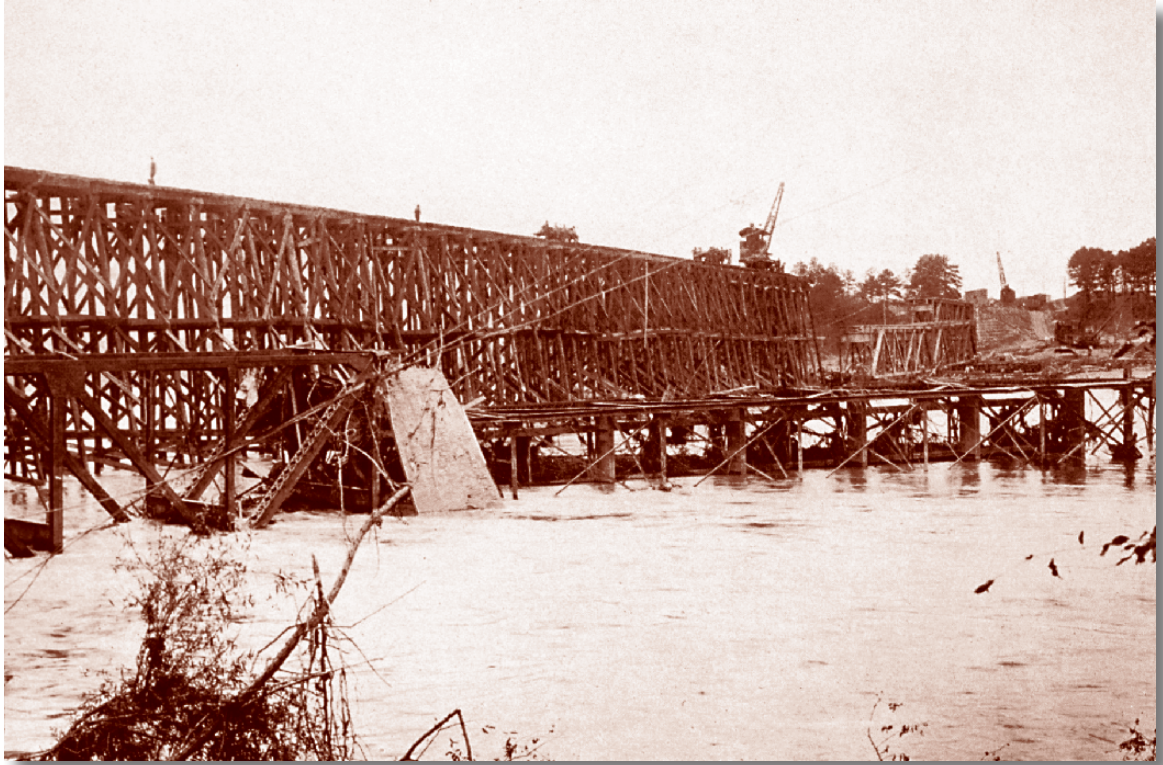
A temporary railroad bridge was built across the Catawba River at Fort Mill, South Carolina, in 1916.
