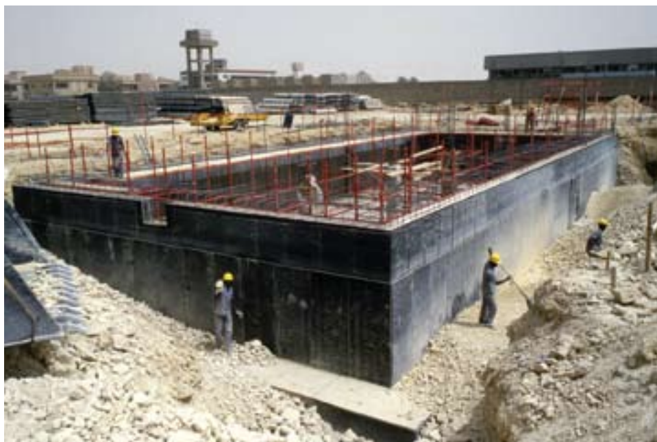
Construction of a potable-water tank for the Royal Saudi Air Force headquarters, Riyadh
