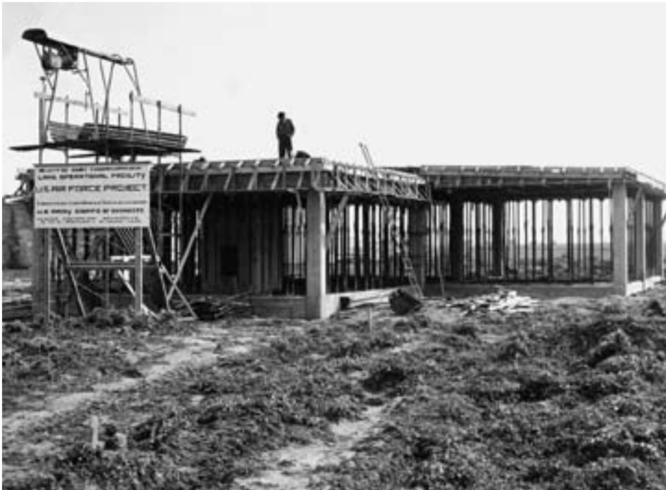
Form for concrete roof under construction for the U.S. Air Force at San Vito, March 1970
