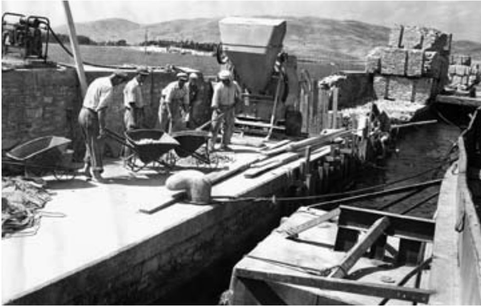
During World War II, the Germans destroyed much of Greece's infrastructure. An American contractor reconstructed an area of the breakwater in Volos Harbor.
