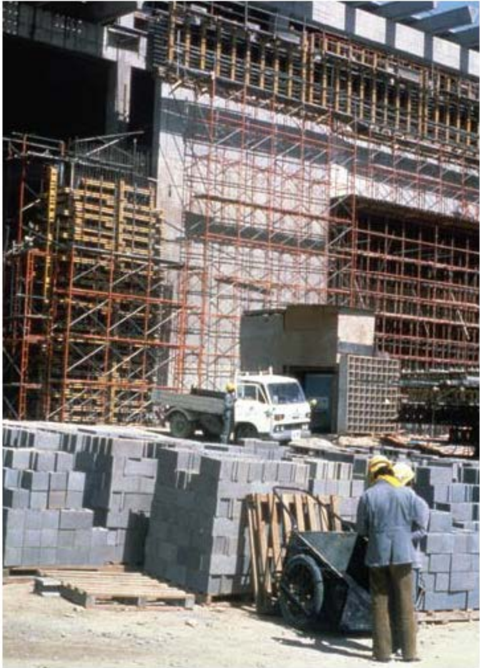
Main entry to the library/administration building under construction at King Abdulaziz Military Academy, early 1980s
