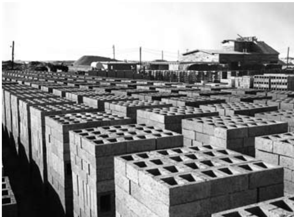
Concrete blocks drying in front of the batch plant at the Dhahran airfield
