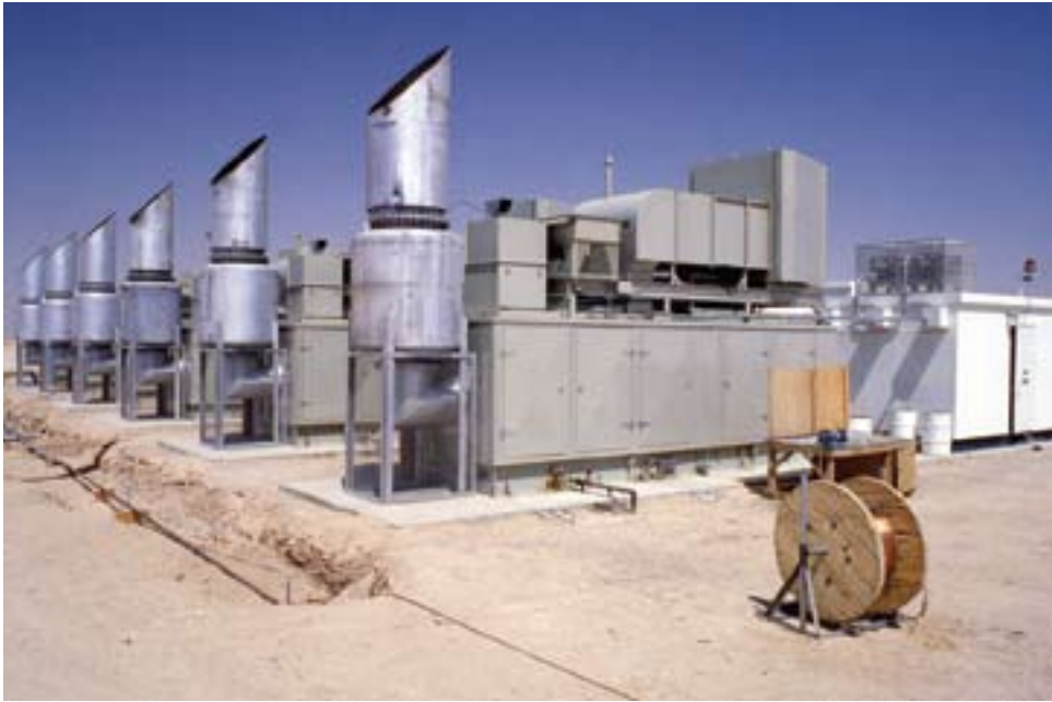
Generator turbines at Hafar al Batin
