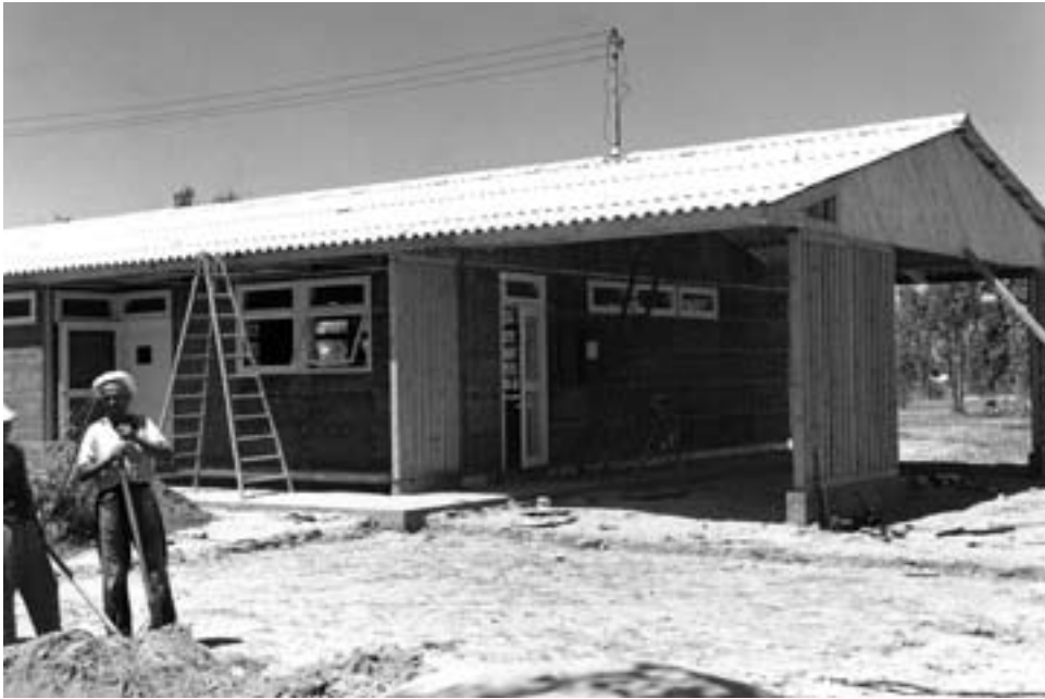
Plans called for forty units of surplus commodity housing with aluminum roofing at Sidi Slimane, shown here in May 1959.
