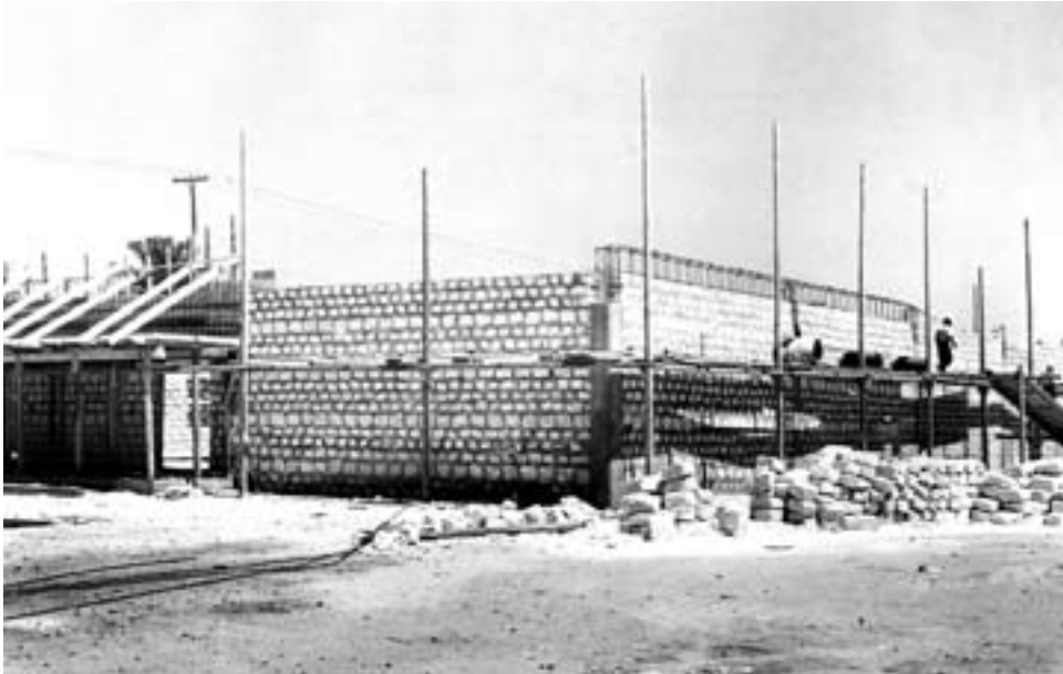
For the communications center, under construction at Wheelus Air Base in August 1951, native limestone blocks were placed to the first bond beam level and reinforced steel was used for a section of the bond beam.
