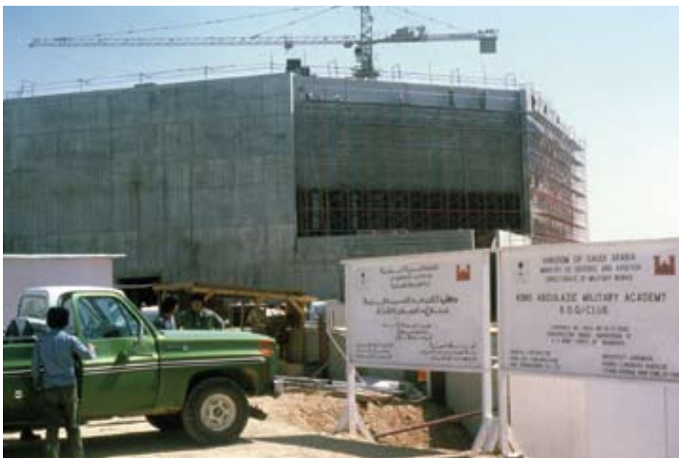
Construction of bachelor officers quarters and club at King Abdulaziz Military Academy, April 1982
