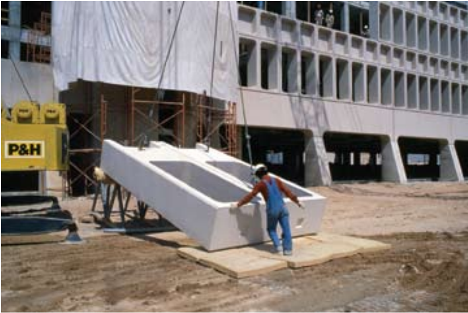
Construction of the Saudi Arabian National Guard headquarters using precast concrete, August 1978
