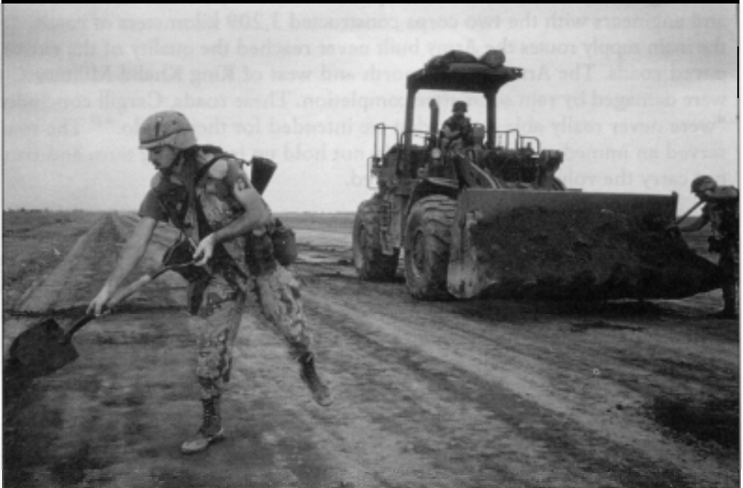
Soldiers and equipment from the 20th Engineer Brigade work on a new road bed. (U.S. Army photo by SSG Martello, 20th Engineer Brigade, Public Affairs Office)
