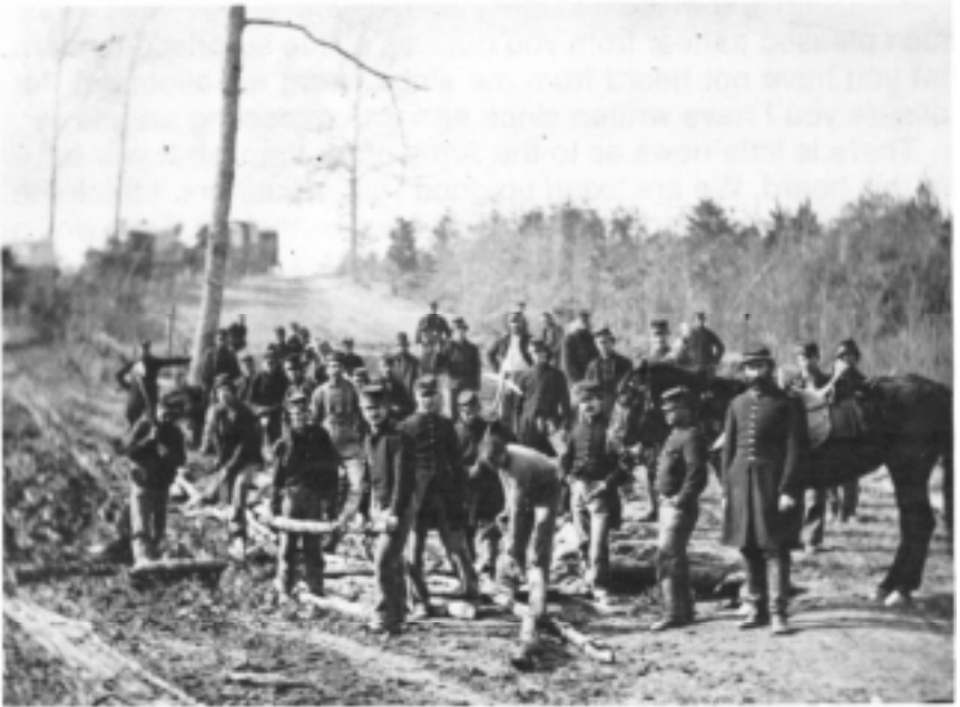
Engineer troops building corduroy road, Richmond, Virginia, June 1862. Library of Congress photograph B8171-656.
