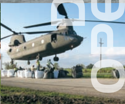
Sandbags weighing 4,000 pounds each are hooked to an Army National Guard CH-47 Chinook helicopter to repair a broken levee near New Orleans after Hurricane Gustav.
