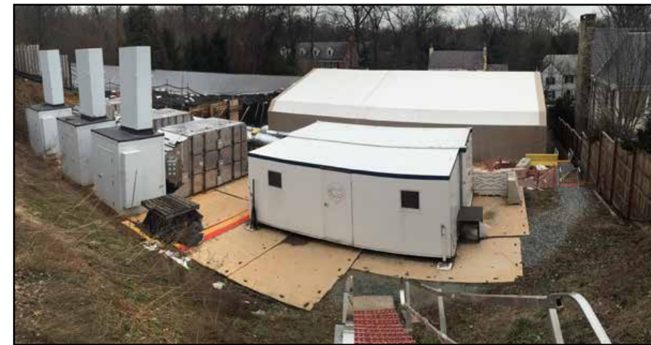
The Engineering Control Structure (the tan tent) and other aspects of the multi-layered approach to public safety USACE had in place during high probability operations at the Glenbrook Road cleanup site are visible among the homes in the Washington, D.C., Spring Valley neighborhood. (Courtesy photo)
