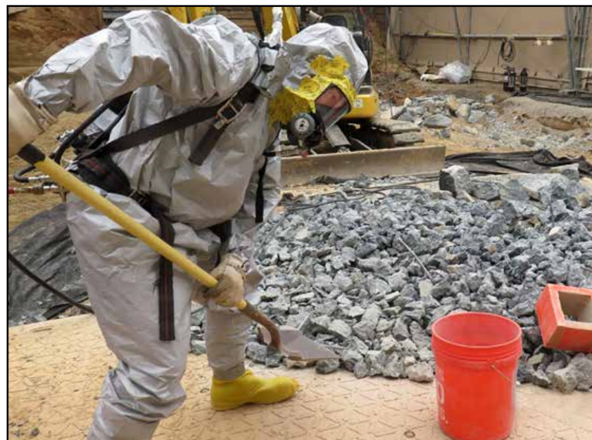
After being broken into small enough pieces to be inspected for contamination, concrete rubble from the basement footers of the house is shoveled into containers to be removed from the site. (Courtesy photo)
