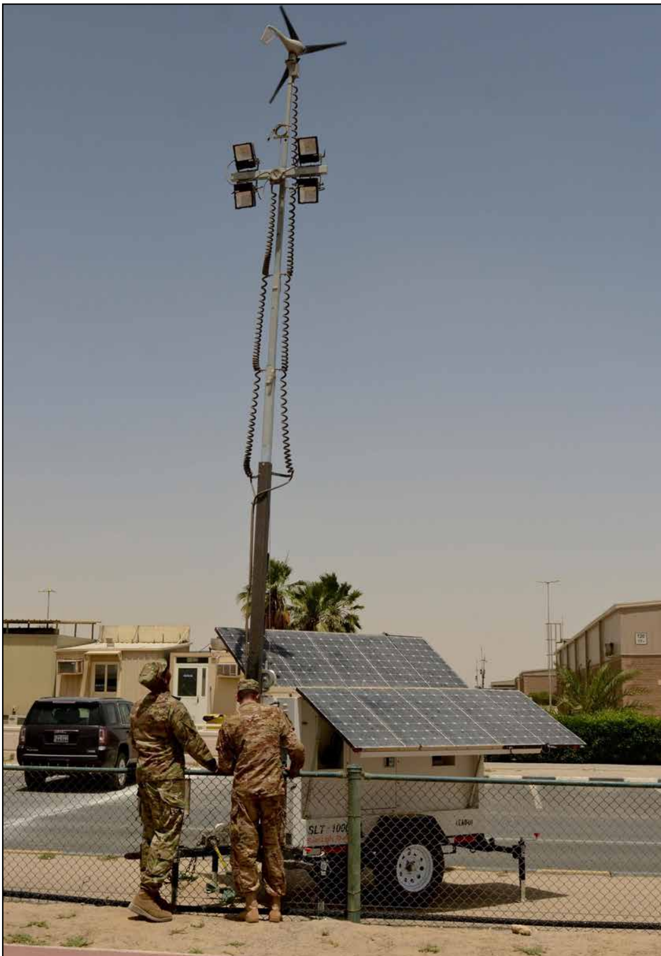
Chief Warrant Officer 3 Weaver Prosper, the U.S. Army Central Command operational energy program manager, and Staff Sgt. Adam Isdale, the noncommissioned officer in charge of the USARCENT forward engineers, inspect a solar-powered light system on Camp Arifjan, Kuwait, May 16.
