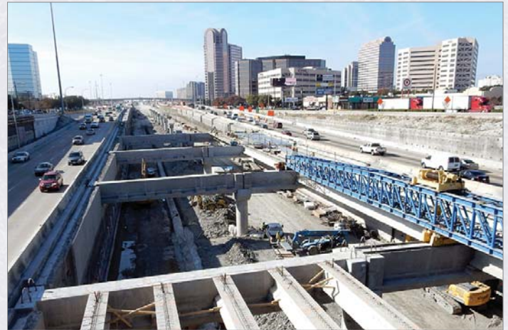
Looking westbound at the construction on the depressed TExpress Lanes on LBJ Express between Preston Road and the Dallas North Tollway
