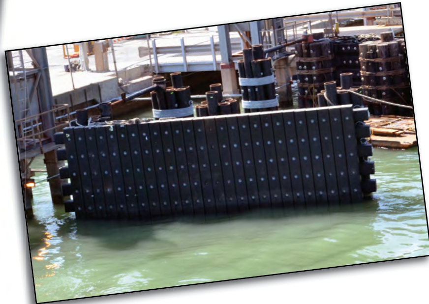
At left, the crane from the Russell Marine positions the pilings for the new composite clusters. Above is one of the recently completed fender walls Port Aransas Ramp 2.
