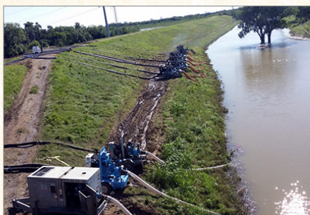
TxDOT crews pumping tens of millions of gallons of water back inside the levees of the Trinity River and off of State Loop 12.
