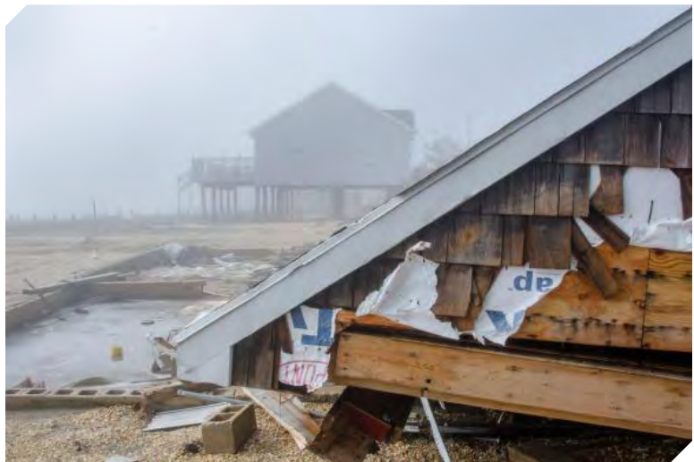
Ocean Gate, N.J., Jan. 30, 2013 -- The home on pilings, in the background, survived Hurricane Sandy with relatively little damage, while its neighbor (foreground) was not as fortunate. Photo by Liz Roll/FEMA
