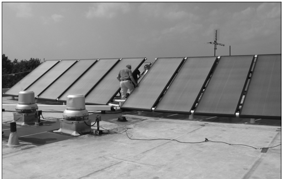
Figure 4: Solar Panels Installed at a SERC Project in Massachusetts
