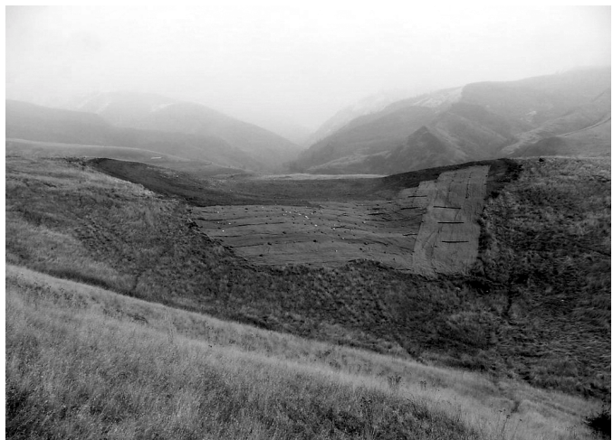
View of the reshaped sand and gravel pit at the White Bird battlefield on November 14, 2000, immediately after reseeded.
