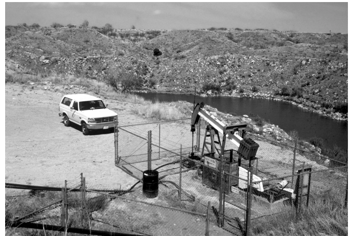
This producing oil well is located near a steep drainage at Lake Meredith National Recreation Area. Stained soils around the pumpjack indicate persistent and recurring leaks. There is no secondary containment to prevent leaks and spills from being released into the environment.
