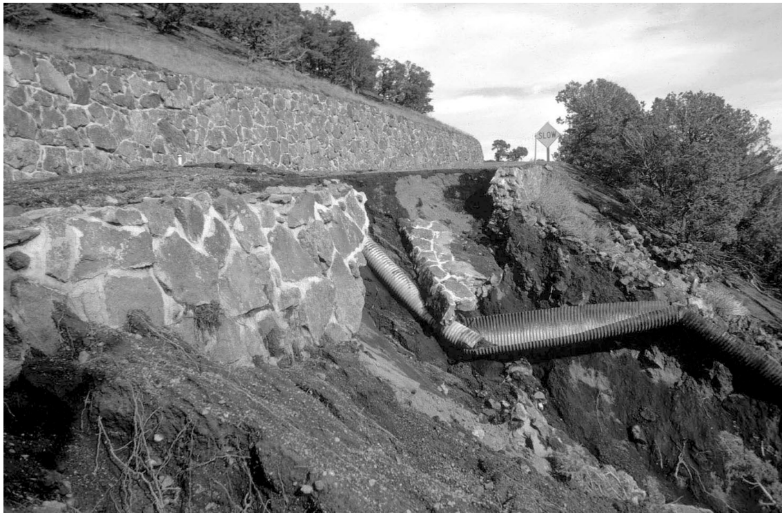
Natural processes were not adequately accommodated during the design of the road at Capulin Volcano National Monument, causing numerous erosional problems. Cooperating with Federal Highway Administration engineers, Division staff provided geomorphic analysis that has led to a plan to reduce impacts to the road and downslope resources.
