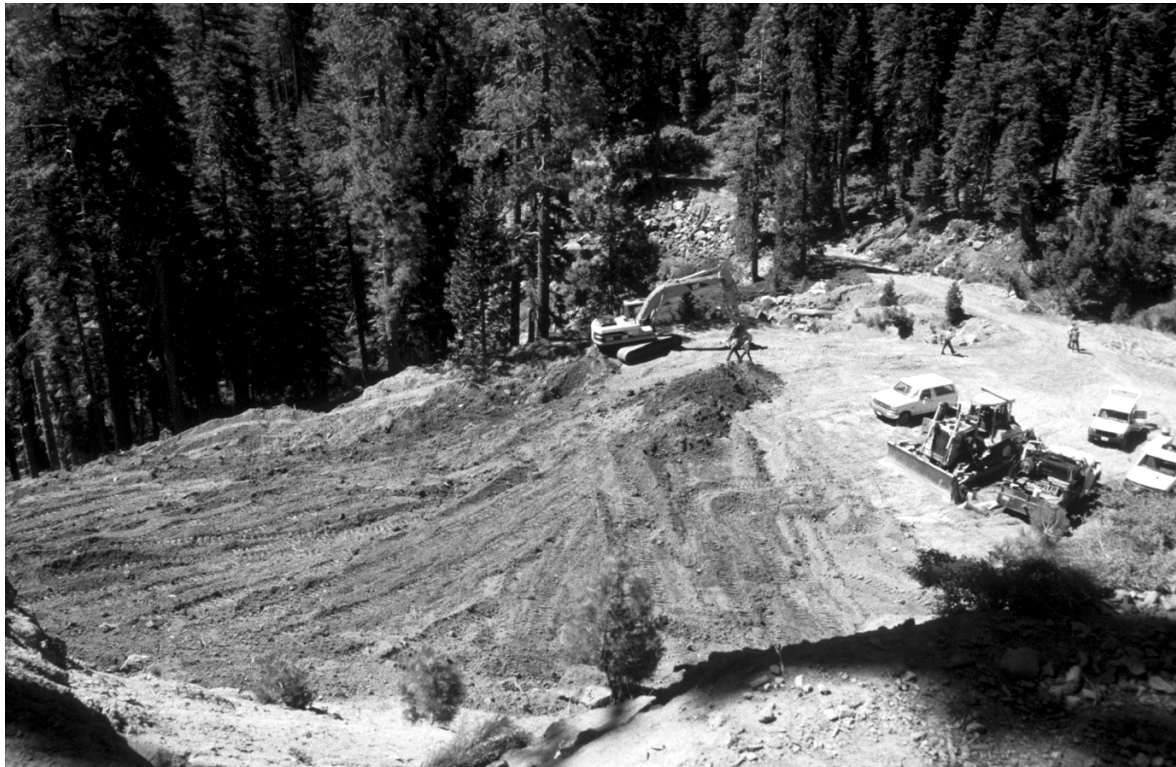
Terminal Geyser geothermal well - After plugging the 4000' deep well to protect nearby thermal features, NPS equipment is beginning to recontour the well pad and access road.
