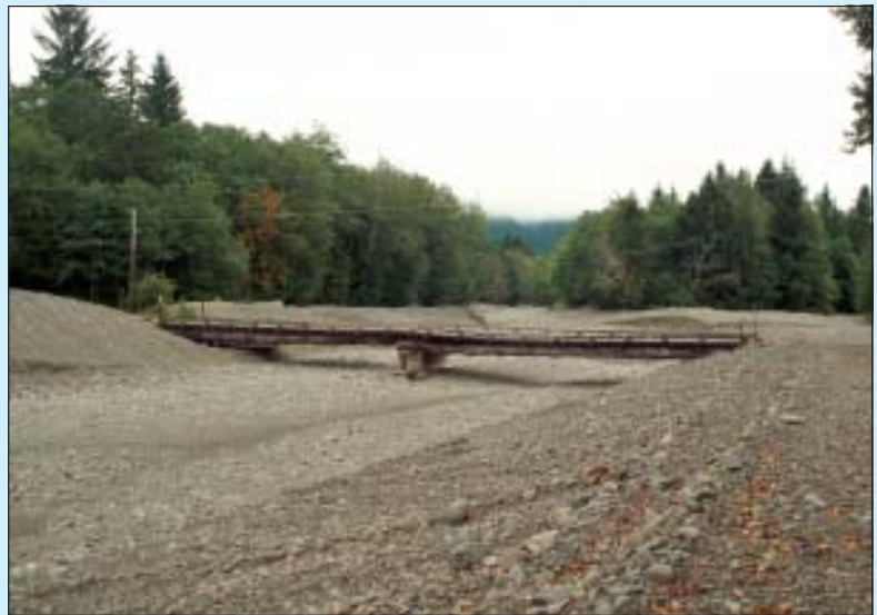
Park Maintenance extracts gravel from Finley Creek Bridge at Olympic National Park to protect the bridge and maintain flows. Photo by Mark Ziegenbein.
