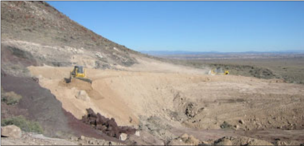
Left: Restoration efforts continue on the JA cone at Petroglyph National Monument. Photo by Deanna Greco.
