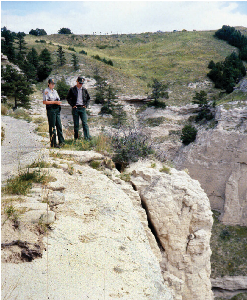
Trailside cracks at Scotts Bluff National Monument, Nebraska provide evidence of ongoing natural bluff retreat and potential rockfall areas.
