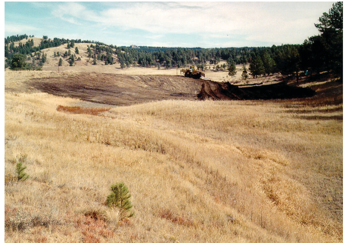
Heavy equipment, similar to that used to construct the dam, is used to reestablish naturally functioning landforms.
