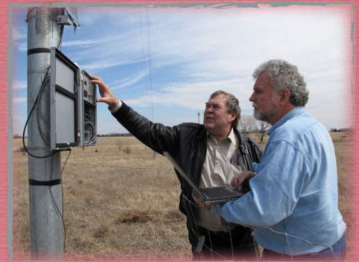
IEED Staff and consultant check wind monitoring equipment for Oklahoma Cherokee Wind Project. Photo: Winter Jojola-Talbert
