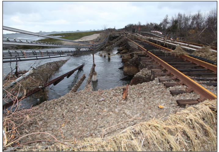
Damage to the Metropolitan Transit Authority Rockaway Line
